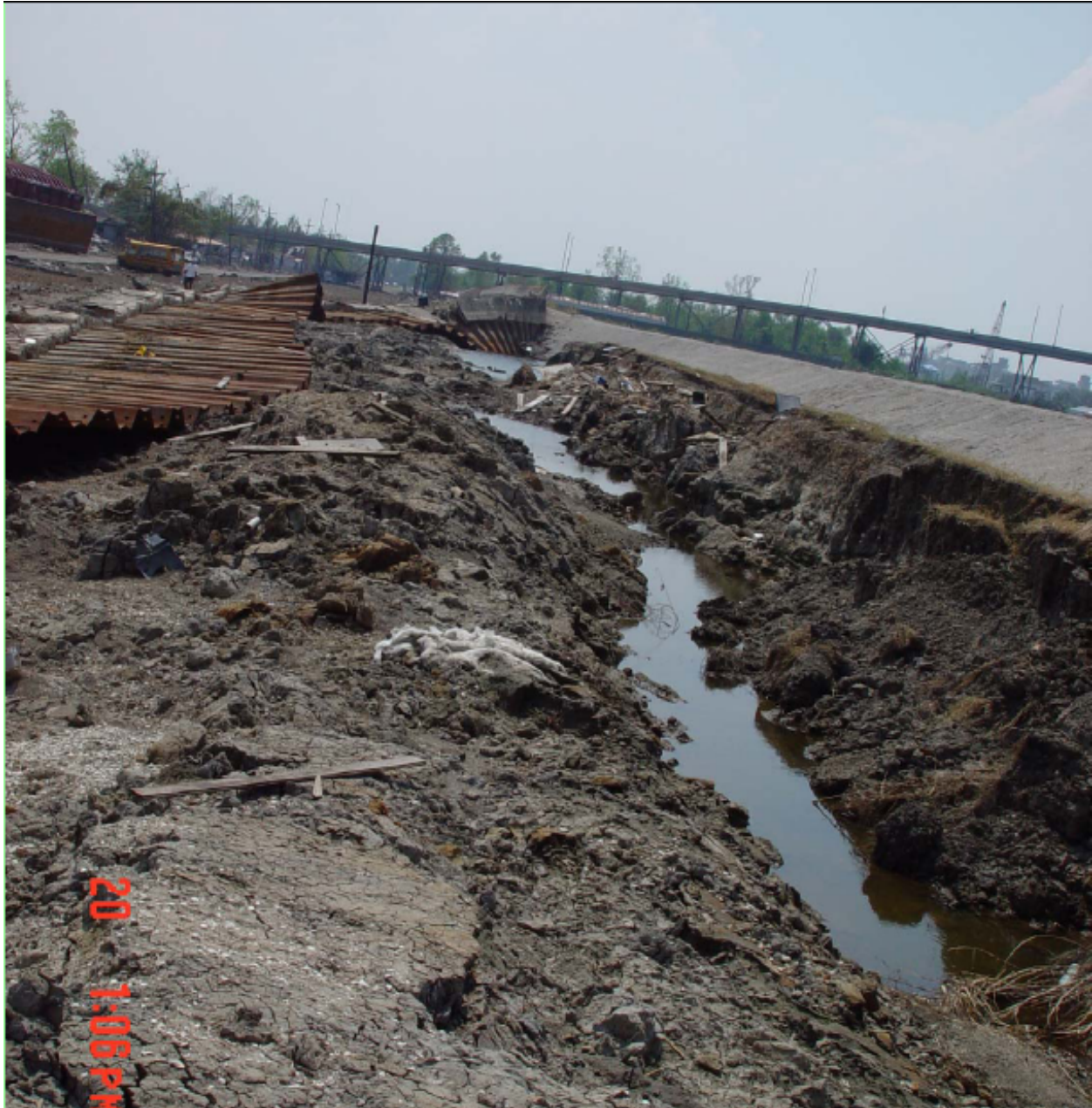
Figure 83. Stage D erosion along the eastern side of the IHNC adjacent to the Lower Ninth Ward.
