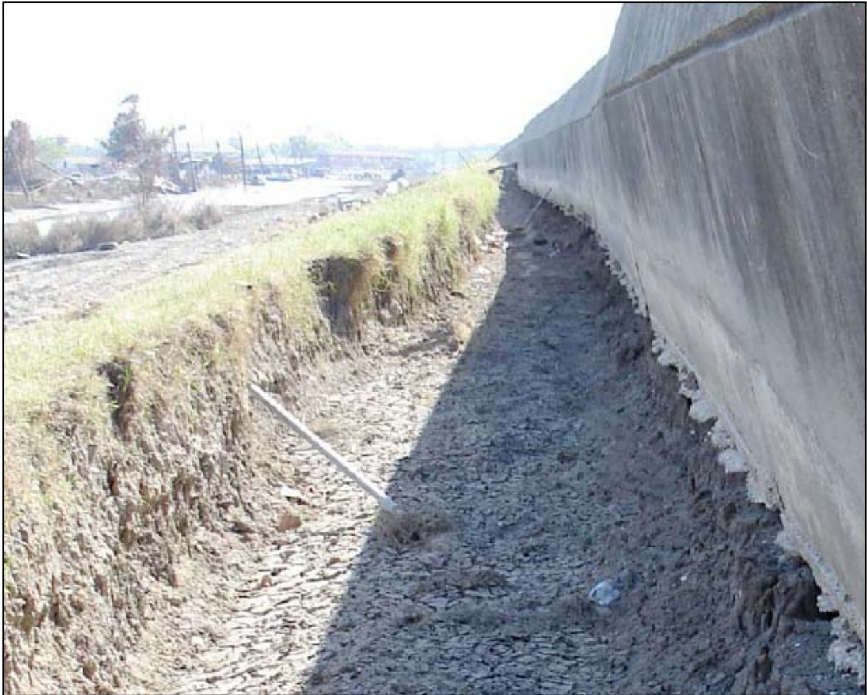
Figure 82. Stage A erosion along the eastern side of the IHNC adjacent to the Lower Ninth Ward.
