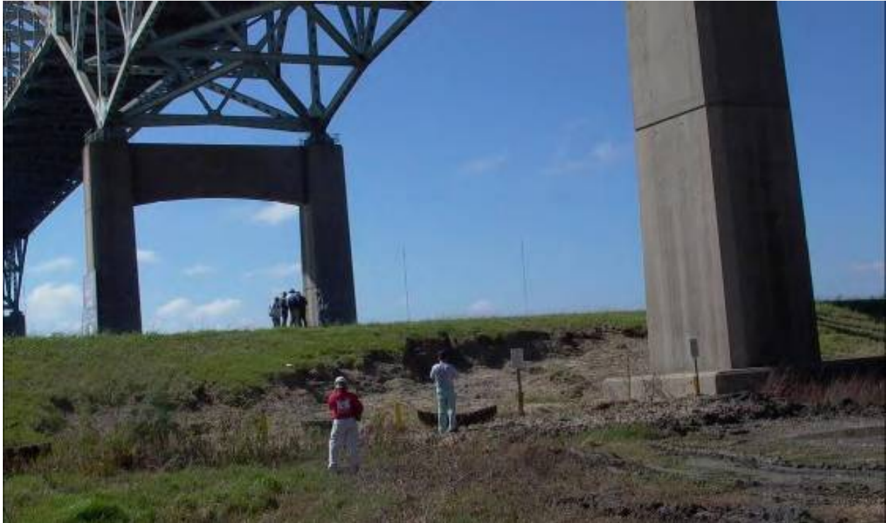
Figure 96. Overtopping of the levee under the Paris Road Bridge adjacent to the Entergy power plant in New Orleans East after the storm.
