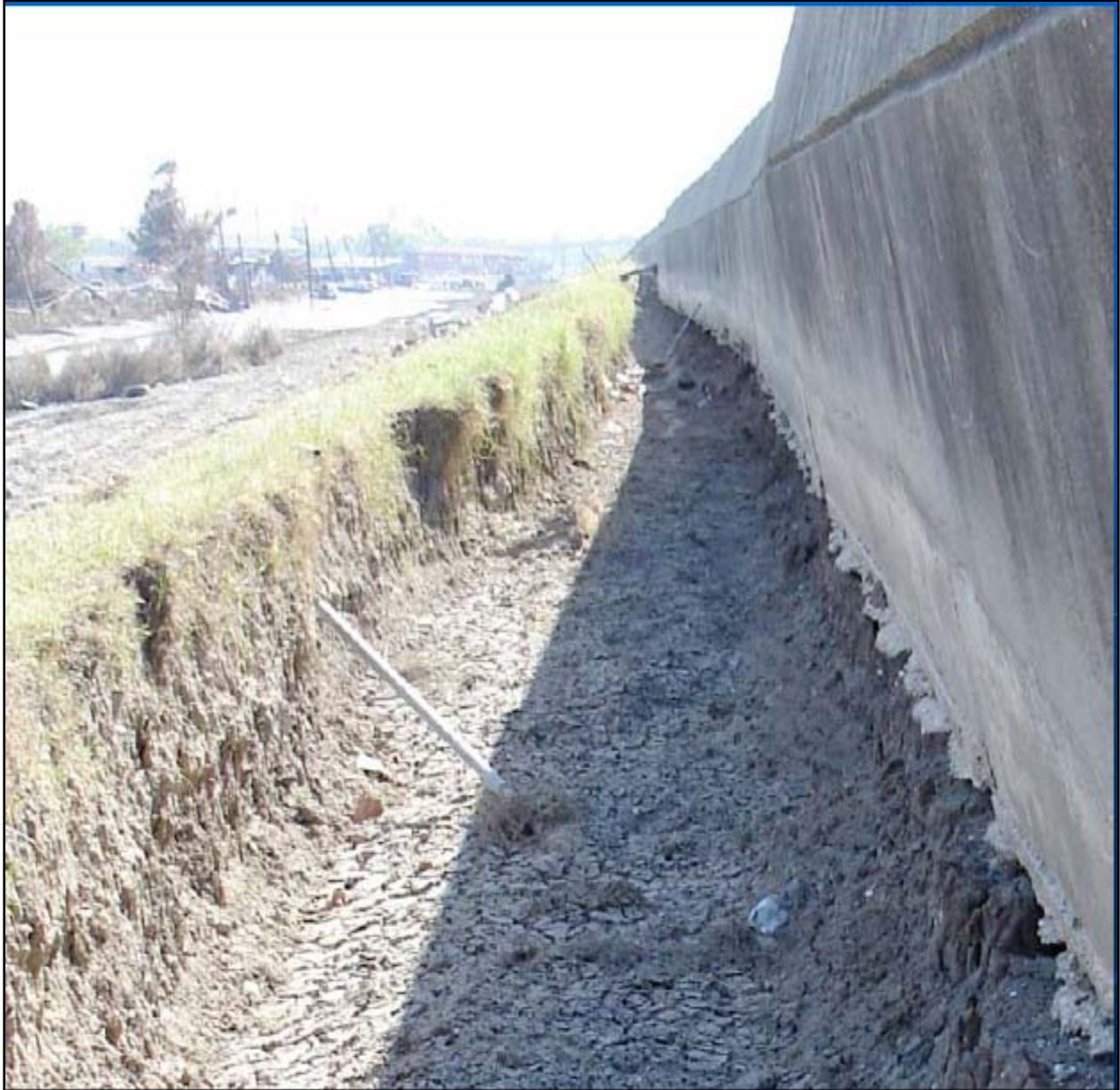
Figure 52. Scour and Erosion on the Protected Side of the IHNC adjacent to the 9th Ward in the vicinity of the south breach.
