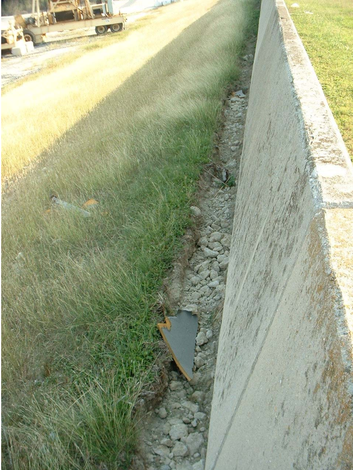
Figure 65b. Post-Katrina photographs of Michoud Canal I-wall showing erosion from overtopping waves.
