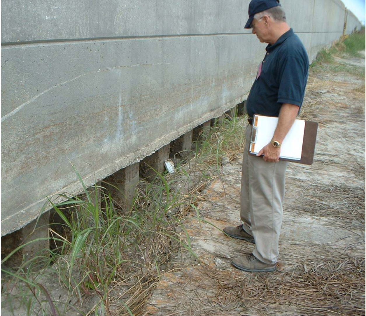
Figure 65a. Post-Katrina photographs of Michoud Canal I-wall at pump station.
