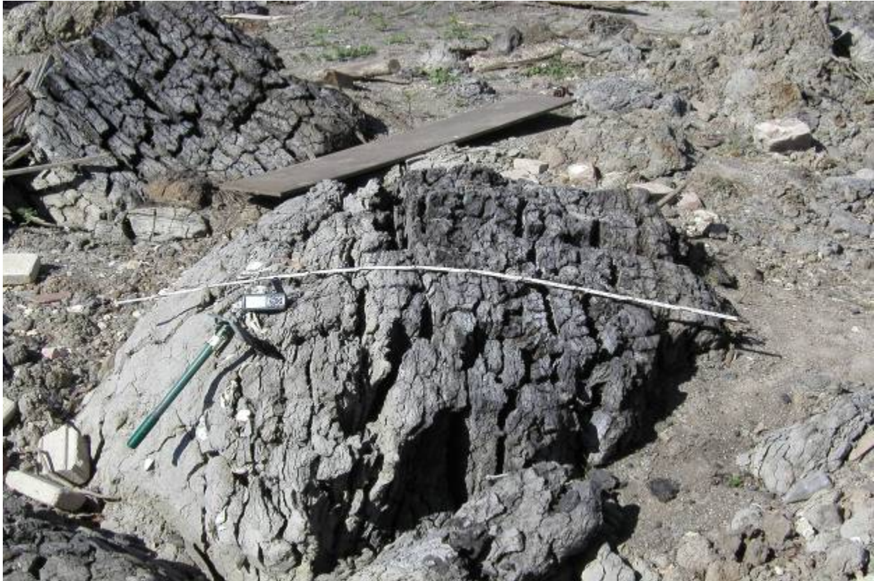
Figure 15. Clay attached to marsh blocks at the 17th Street Canal breach.
