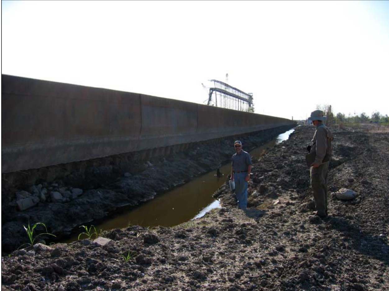
Figure 77. Scour trench on the protected side of the Citrus Back Levee I-wall. (Figure 7.14, NSF-Berkeley report (ILIT Final Report, 31 July 2006).)
