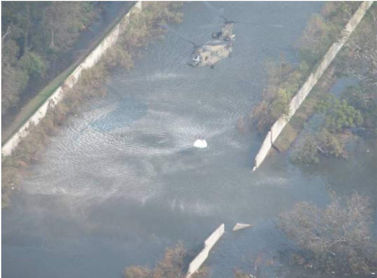
Figure 35. South breach, London Avenue Canal.
