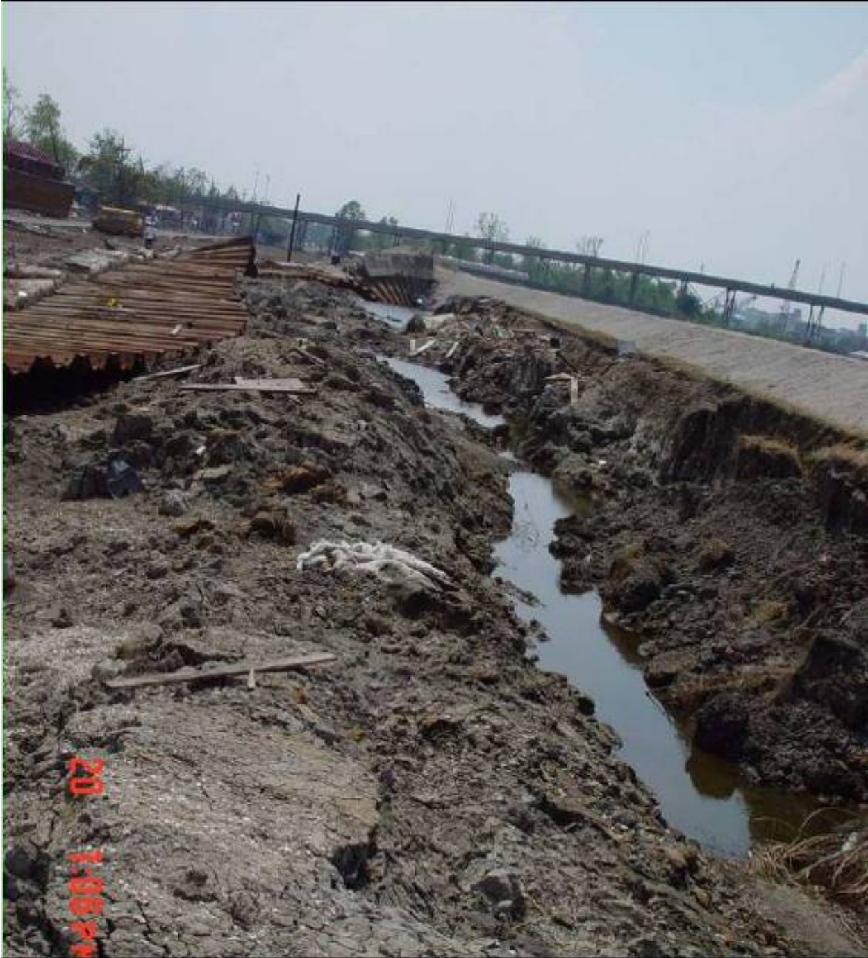
Figure 53. Scour and erosion leading to the failure of the I-wall on the IHNC adjacent the south breach (9th Ward).
