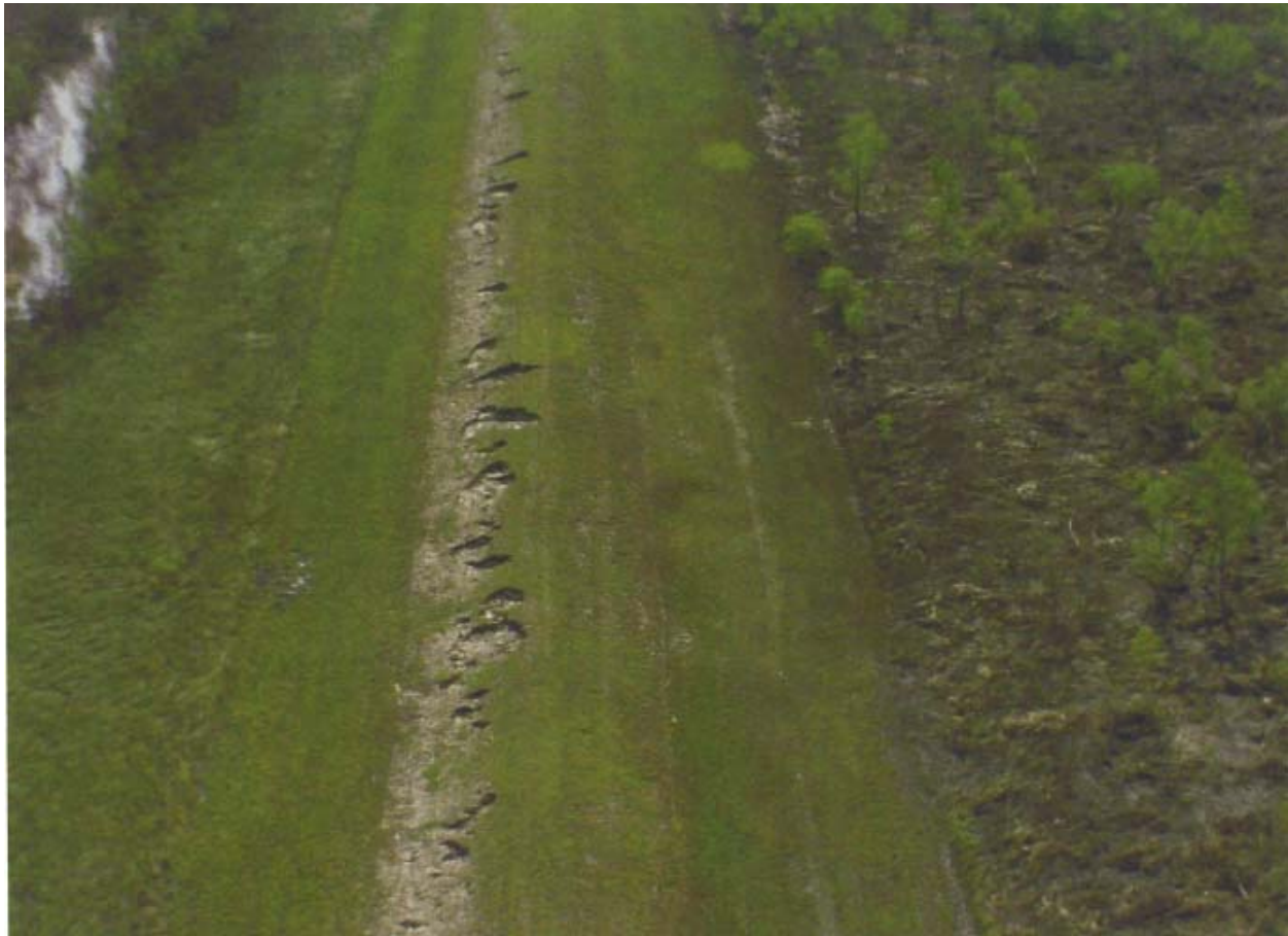
Figure 68. Front side levee erosion along the Mississippi River Gulf Outlet.
