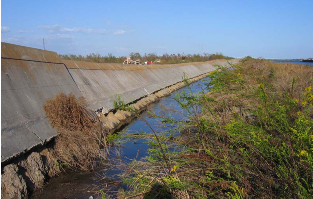
Figure 79. Deflection and tilting of the Citrus Back Levee I-wall.
