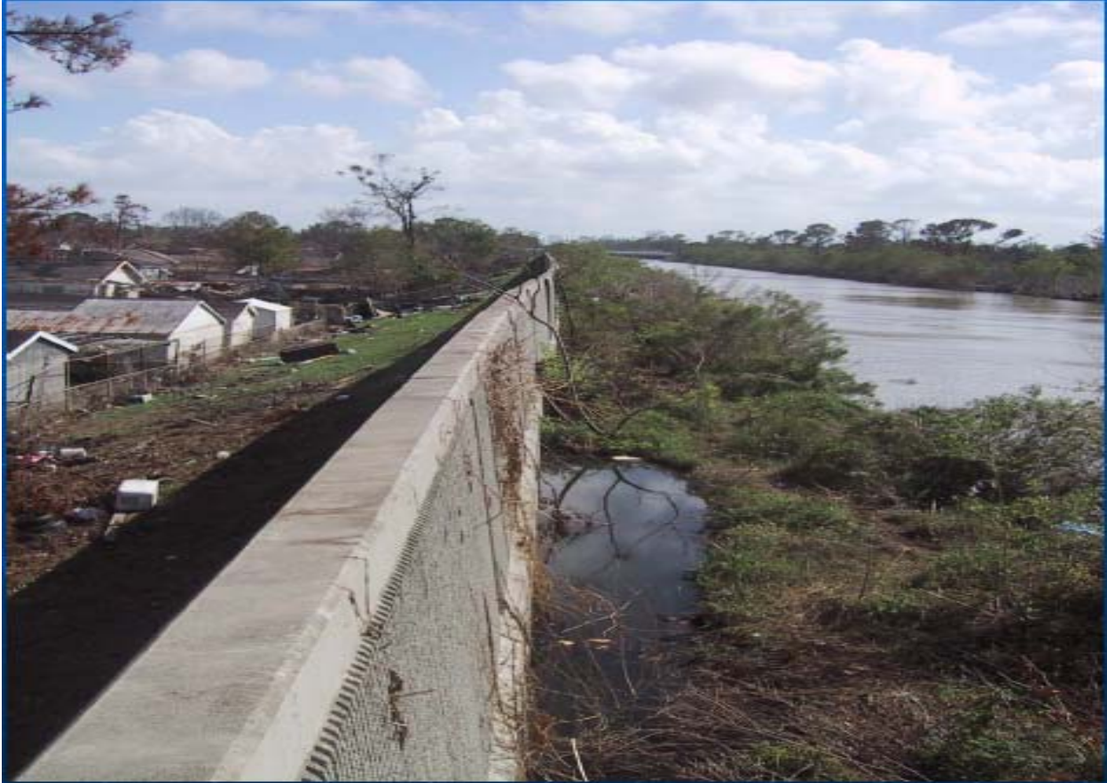
Figure 38. Tilted I-wall opposite the north breach on the London Avenue Canal.
