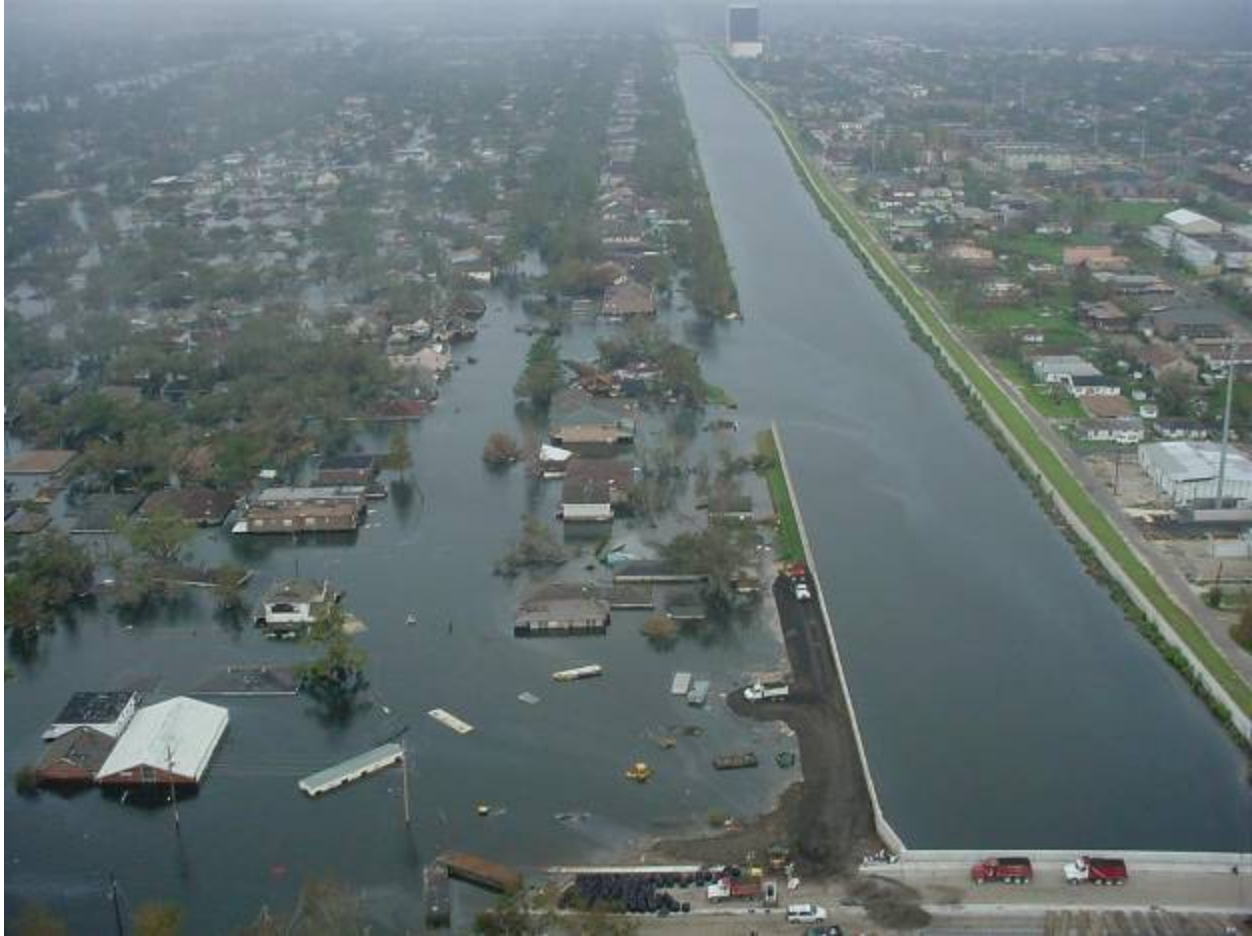
Figure 9. Aerial photograph of the 17th Street Canal breach looking south from the Old Hammond Road Bridge.
