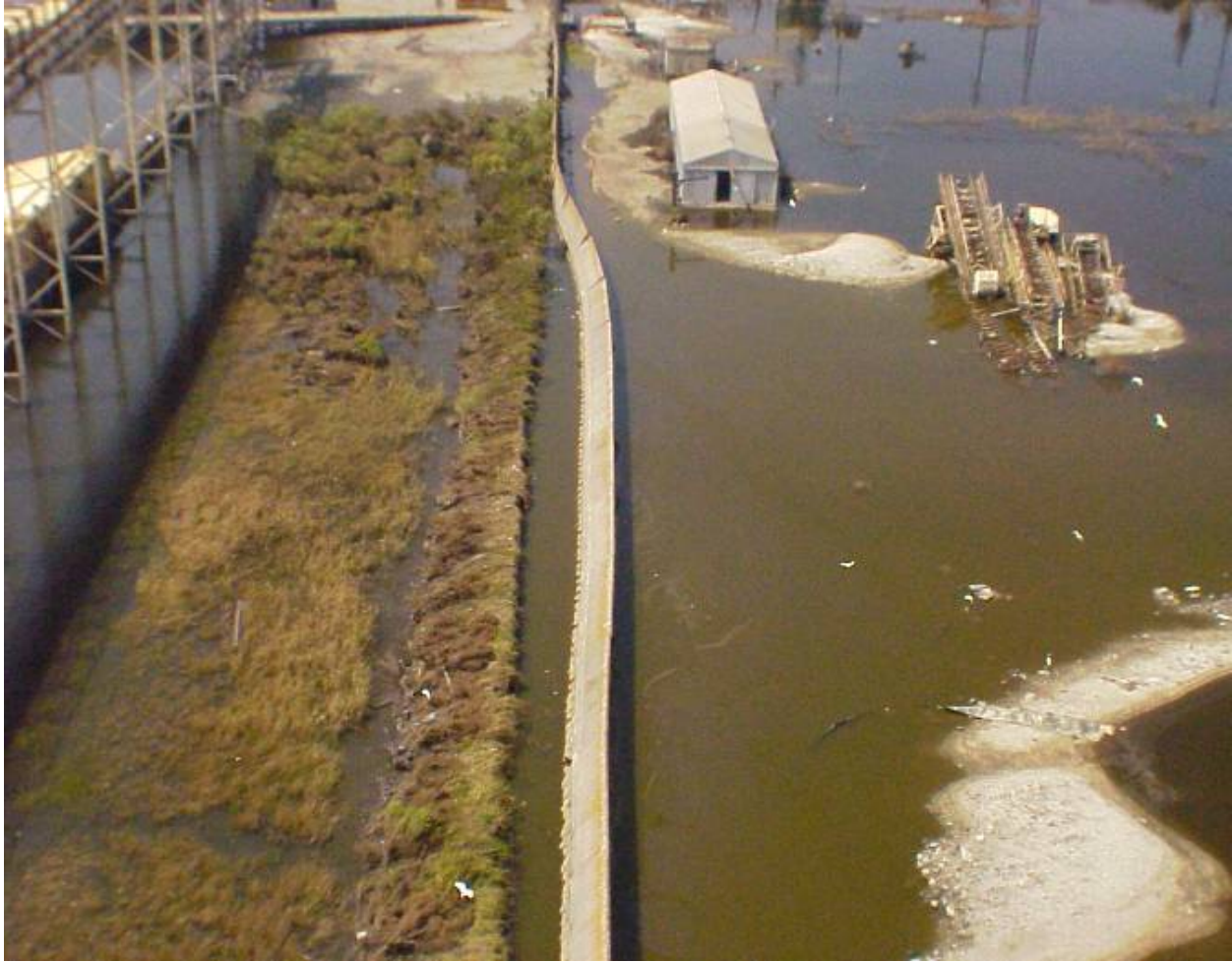
Figure 76. Aerial photo showing the deflection and tilting of the Citrus Back Levee I-wall.
