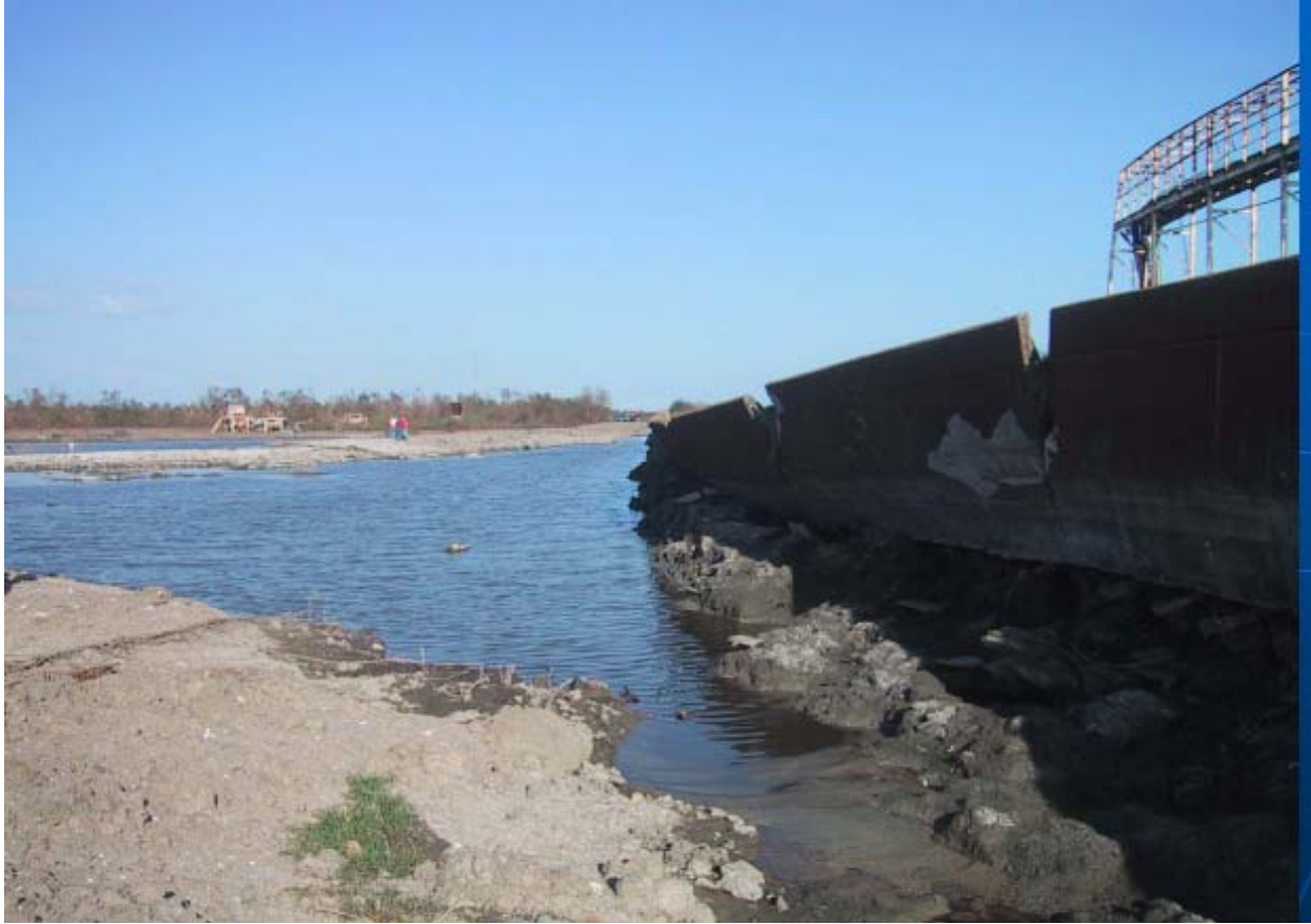
Figure 78. Another section of the Citrus Back Levee I-wall showing erosion of the levee, lateral deflection, and tilting from overtopping.
