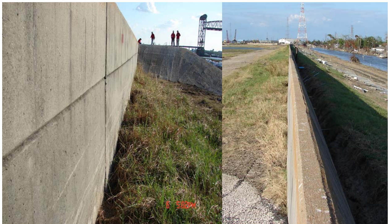
Figure 55. IHNC East Bank – south breach – wall movement.
