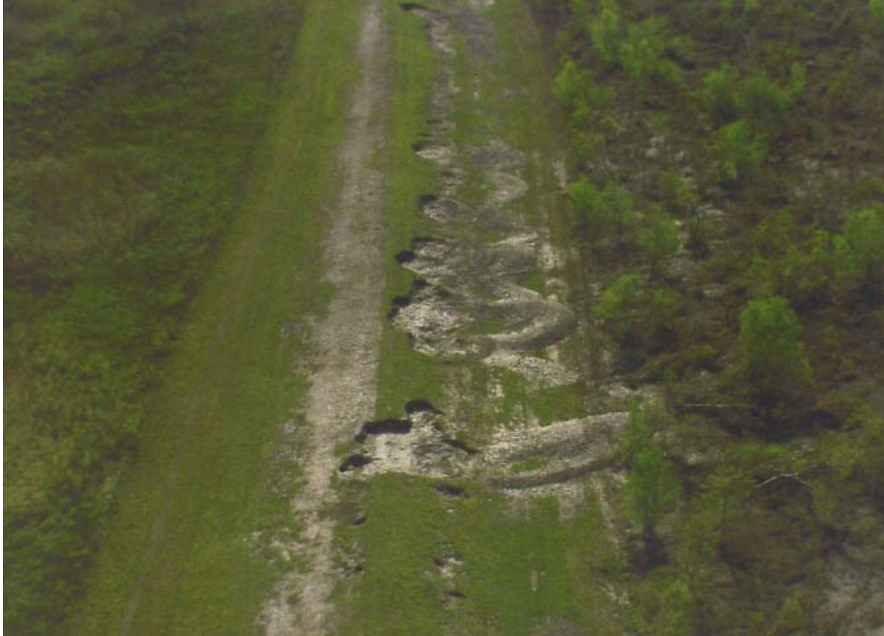
Figure 73. Four stages of progressive erosion.
