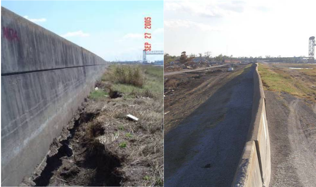
Figure 56. IHNC East Bank – north breach – wall movement.
