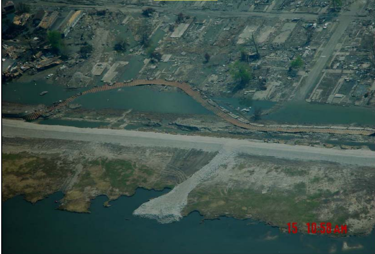
Figure 81. Displaced floodwall along the eastern side of the IHNC adjacent to the Lower Ninth Ward.
