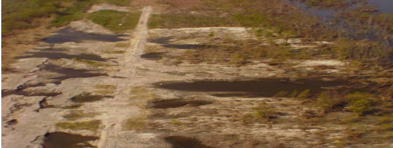
Figure 17. Example of levee along New Orleans East, GIWW, breaching from overtopping and scour of erodible materials.
