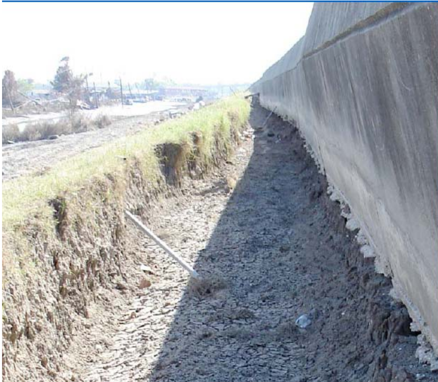
Figure 22. Example of breach along IHNC (east side) from overtopping and scour (top) and scour behind adjacent section that did not fail (bottom).
