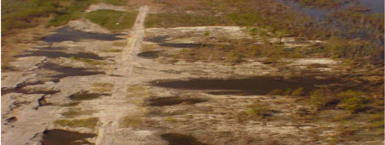
Figure 17. Example of levee along New Orleans East, GIWW, breaching from overtopping and scour of erodible materials.
