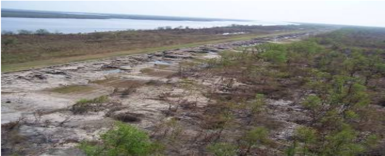
Figure 18. Example of levee breach along MRGO from overtopping and scour of erodible materials.
