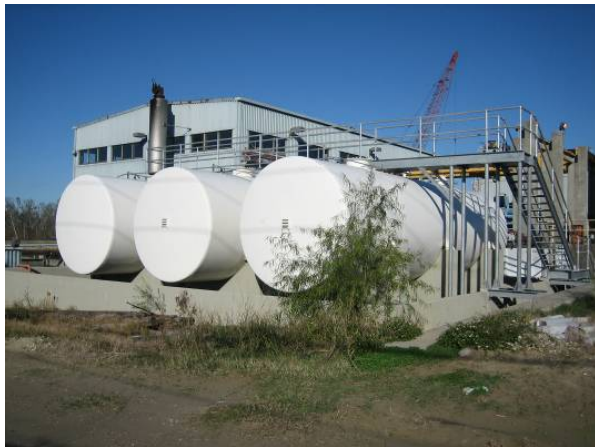
After Hurricane Katrina: View from the side
