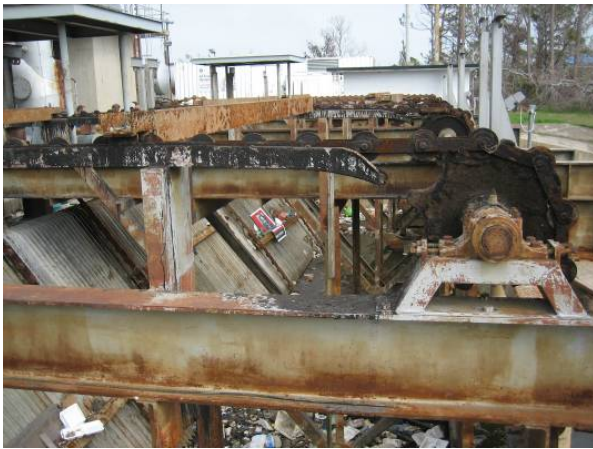
After Hurricane Katrina: View from the discharge
