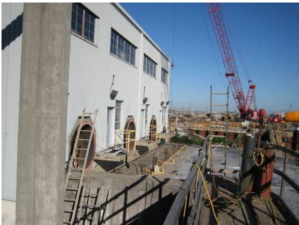
After Hurricane Katrina: View from the discharge
