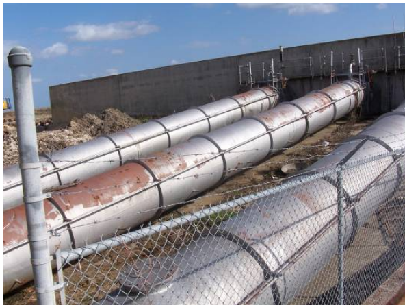
After Hurricane Katrina: View from the discharge
