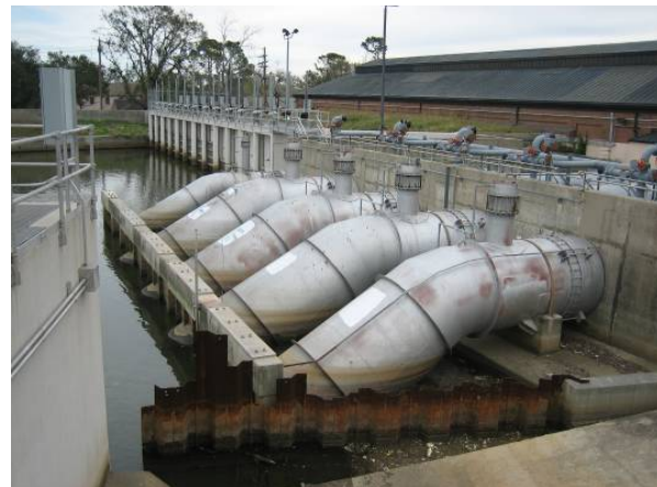
After Hurricane Katrina: View from the discharge
