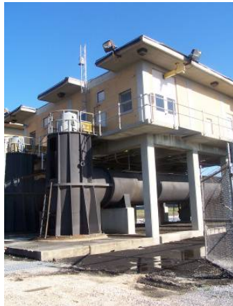
After Hurricane Katrina: View from the side
