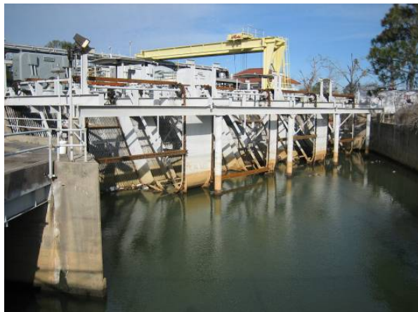
After Hurricane Katrina: View from the discharge
