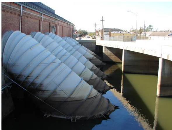
After Hurricane Katrina: View from the discharge
