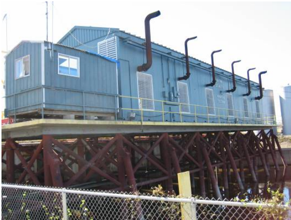
After Hurricane Katrina: View from the discharge
