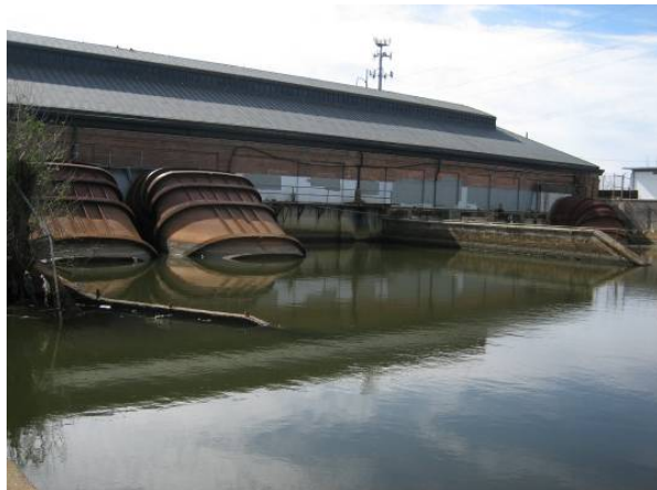
After Hurricane Katrina: View from the discharge
