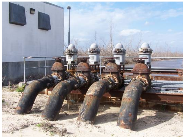
After Hurricane Katrina: View from the discharge
