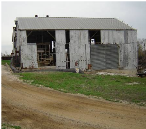
After Hurricane Katrina: View from the inlet canal
