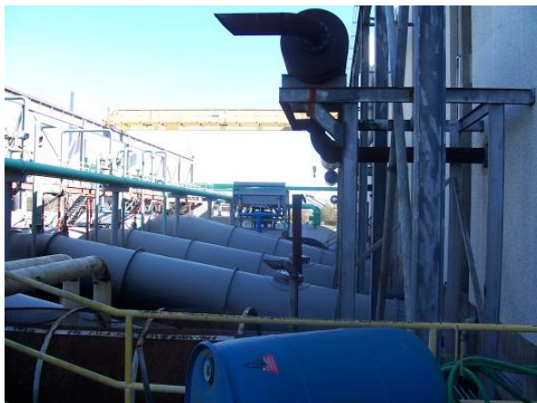
After Hurricane Katrina: View from the discharge
