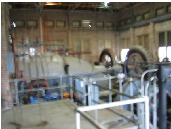
After Hurricane Katrina: View inside the station
