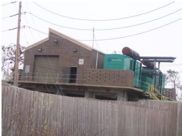
After Hurricane Katrina: View from the side
