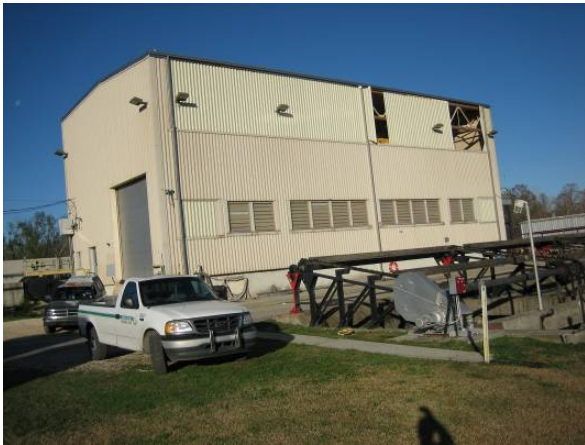
After Hurricane Katrina: View from the intake canal
