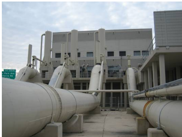
After Hurricane Katrina: View from the discharge
