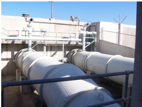
After Hurricane Katrina: View from the discharge
