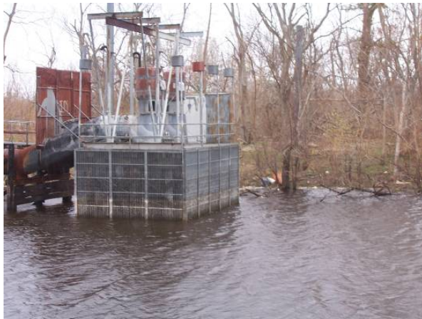
After Hurricane Katrina: View of the station
