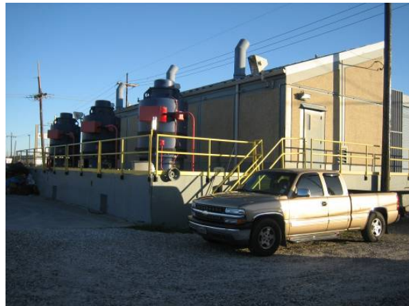
After Hurricane Katrina: View from the discharge
