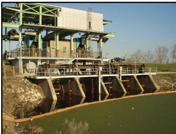
After Hurricane Katrina: View from the inlet canal
