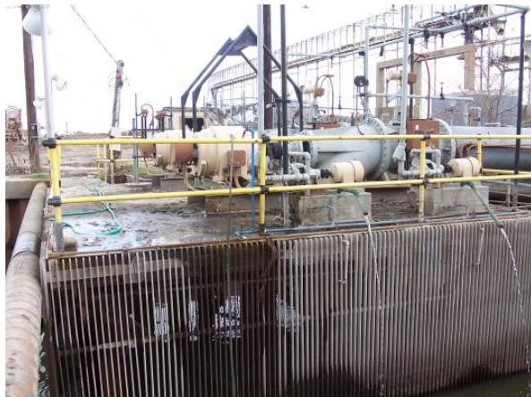
After Hurricane Katrina: View from the discharge
