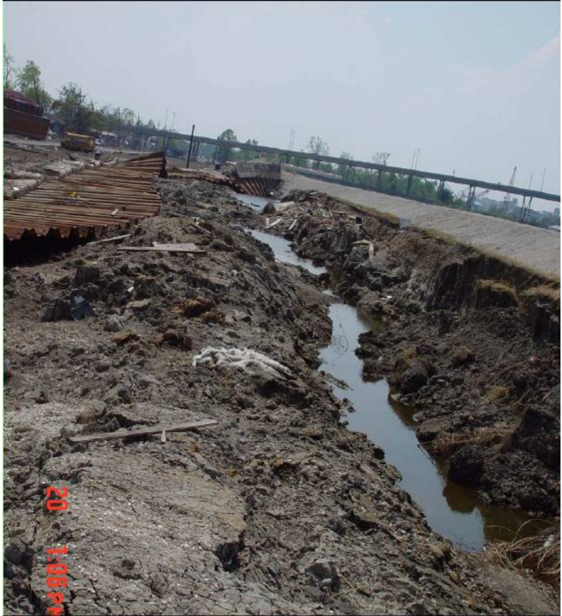
Figure 5. Scour and erosion leading to the failure of the I-wall on the IHNC adjacent the south breach (9 th Ward).
