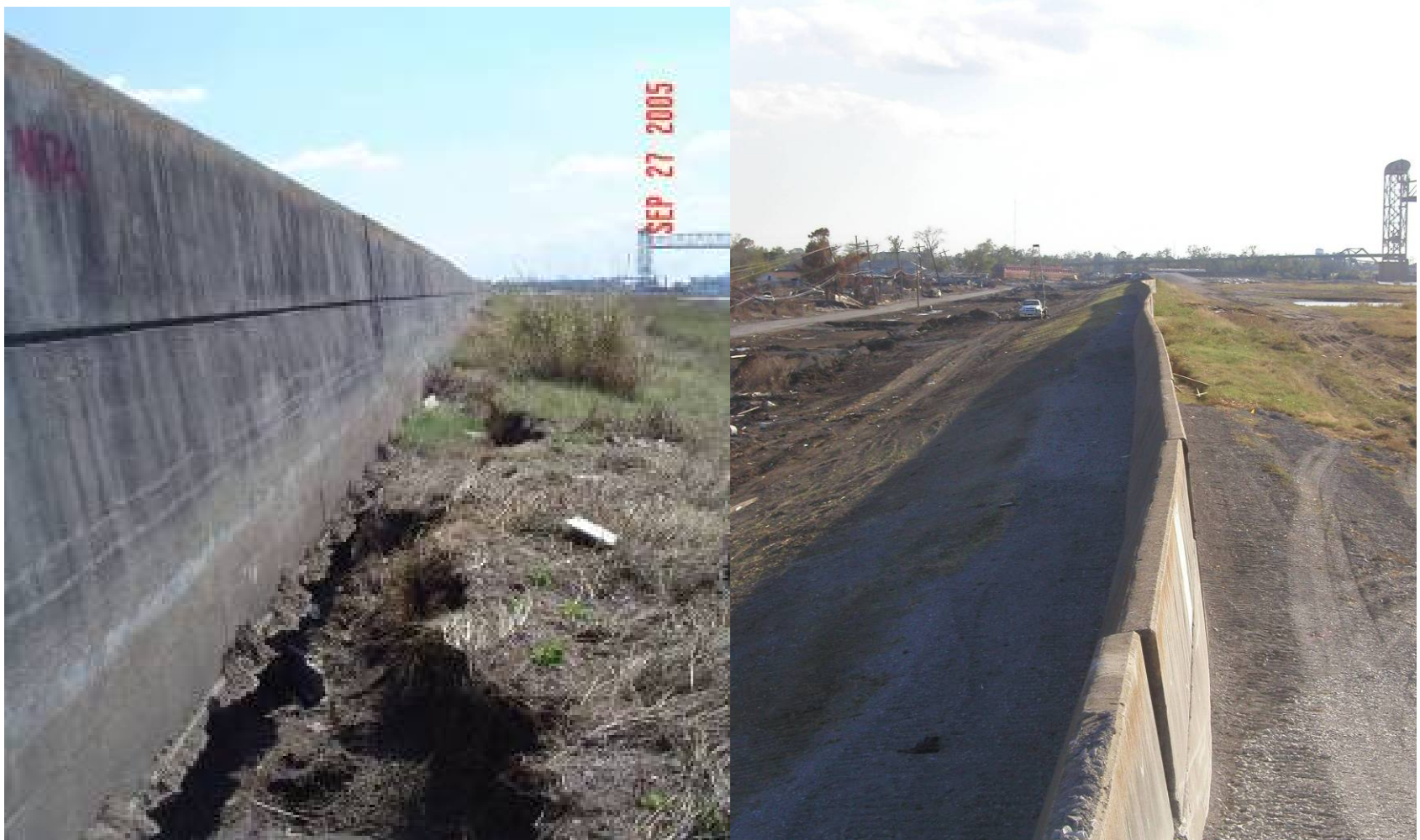
Figure 7. IHNC East Bank – North Breach – Wall movement (View looking south)
