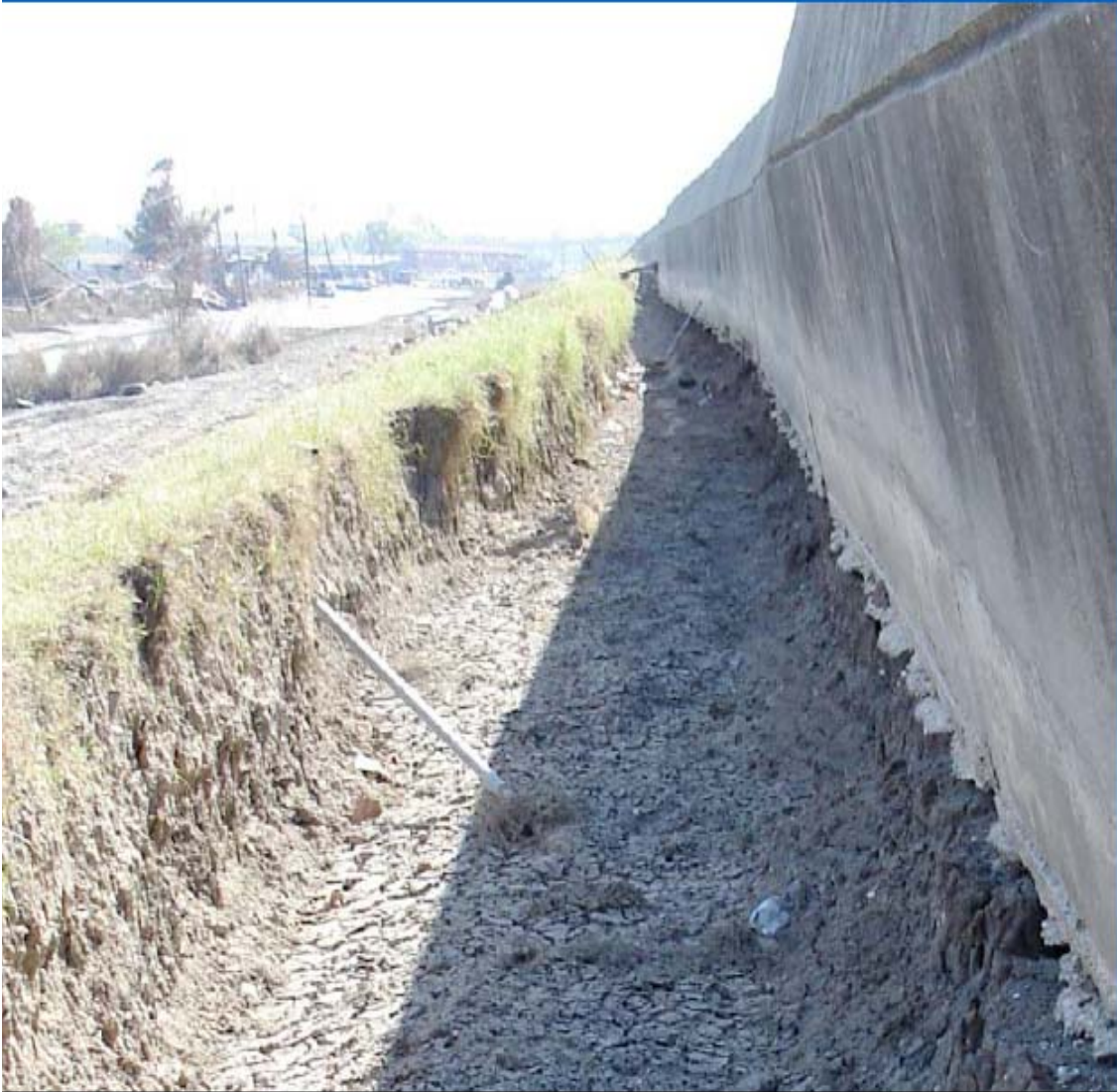
Figure 4. Scour and erosion on the protected side of the IHNC adjacent to the 9 th Ward in the vicinity of the south breach.
