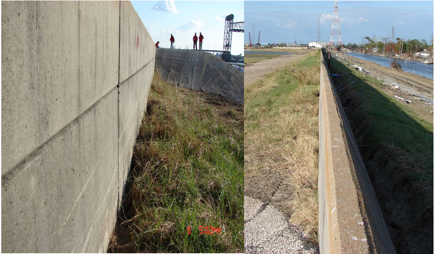
Figure 6. IHNC East Bank – South Breach – Wall movement.
