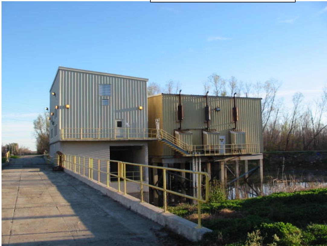
DESTRAHAN #1 PUMP STATION
