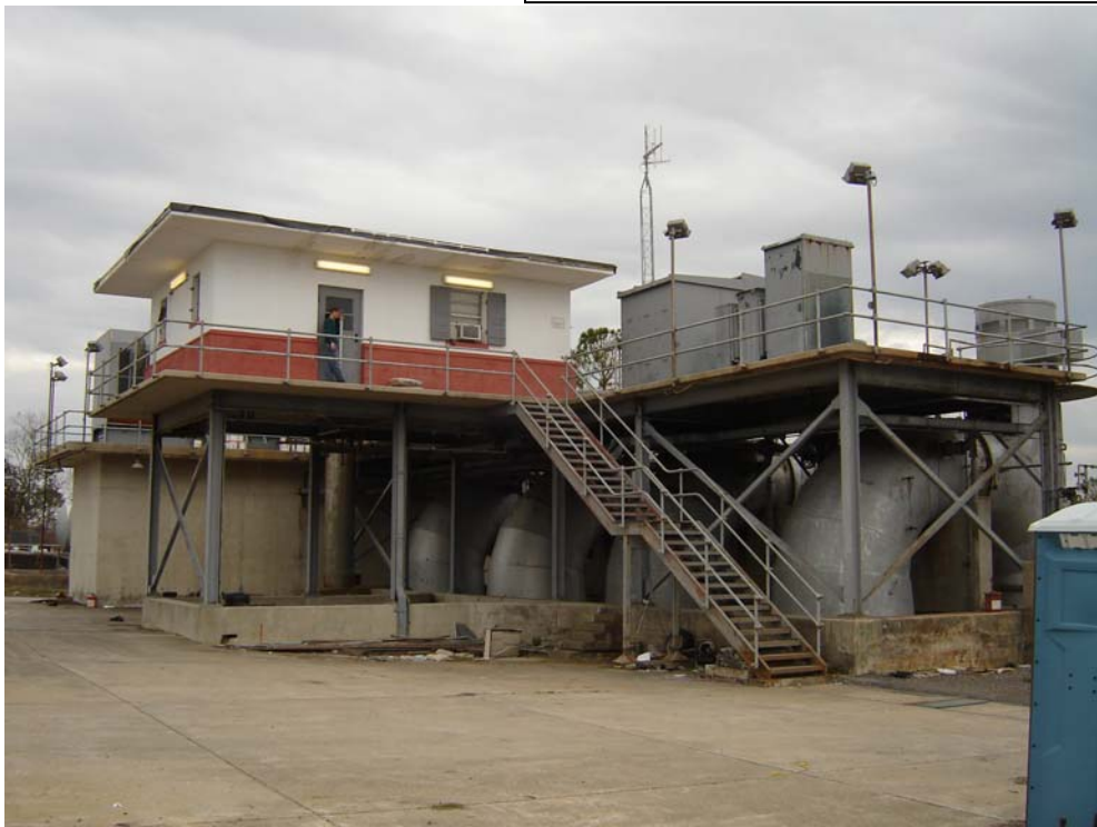
ST. CHARLES OP #16 PUMP STATION
