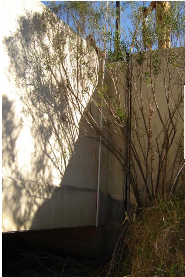
Low Chord Orleans4 #1 East 2.754 feet NAVD88 2004.65 Field Book 060854 Robert E. Lee Boulevard
