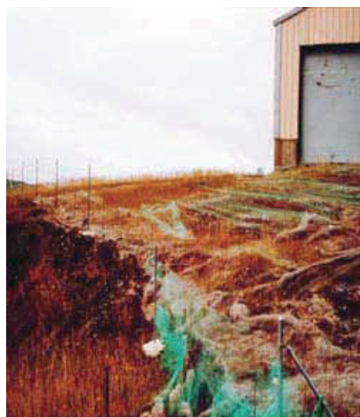
Figure 91: The plastic web or backing has created traps that have ensnared birds and fish - the use of this product should be carefully considered and based on true need and area of use, considering potential consequences.
