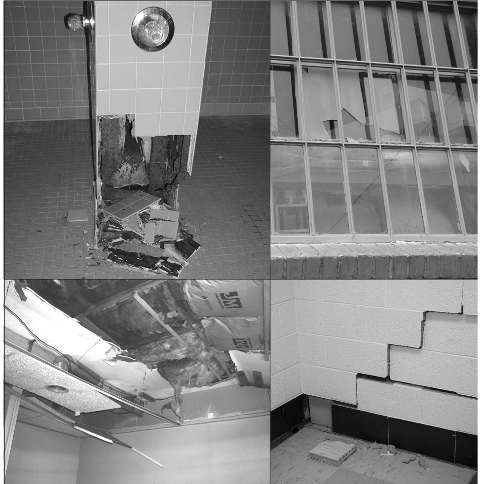
Figure 7: Examples of Damage at Various Reserve Component Facilities
