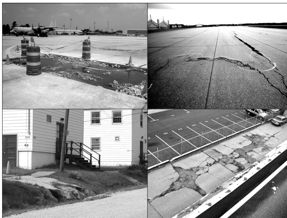
Figure 6: Examples of Deteriorated Ramp, Runway, and Driveways at Various Reserve Component Locations
