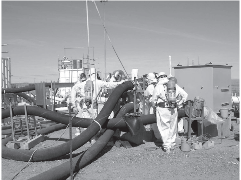
Figure 2: Workers Changing Out Equipment at the Tank Farms at the Hanford Site, a Hazard Category 2 Facility
