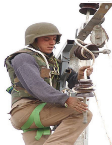
Deployed Army Civilian works to set up Perimeter Lighting system in Taji Iraq. Photo courtesy of USACE Gulf Region Division
