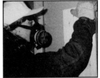
Wear protective clothing and a respirator when removing walls that may contain lead.
