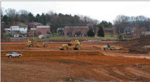
Construction of soccer fields at the Avtex Fibers site in Front Royal, Virginia. Source: EPA
