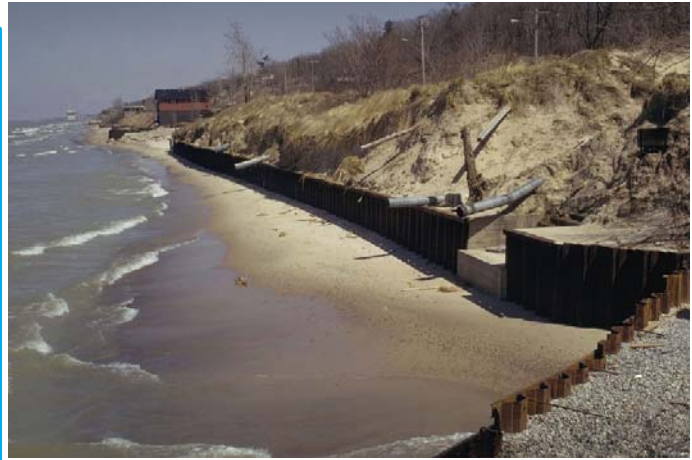
Erosion Along Developed Indiana Shoreline of Lake Michigan
