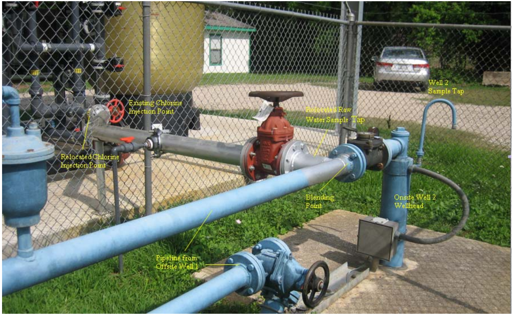
Figure 4-12. Photograph of Piping, Sample Taps, and Chlorine Injection Point Prior to Treatment System
