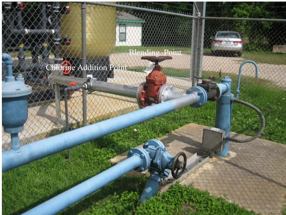
Figure 4-1. Preexisting Chlorine Addition Point and Wells 1 and 2 Blending Point
