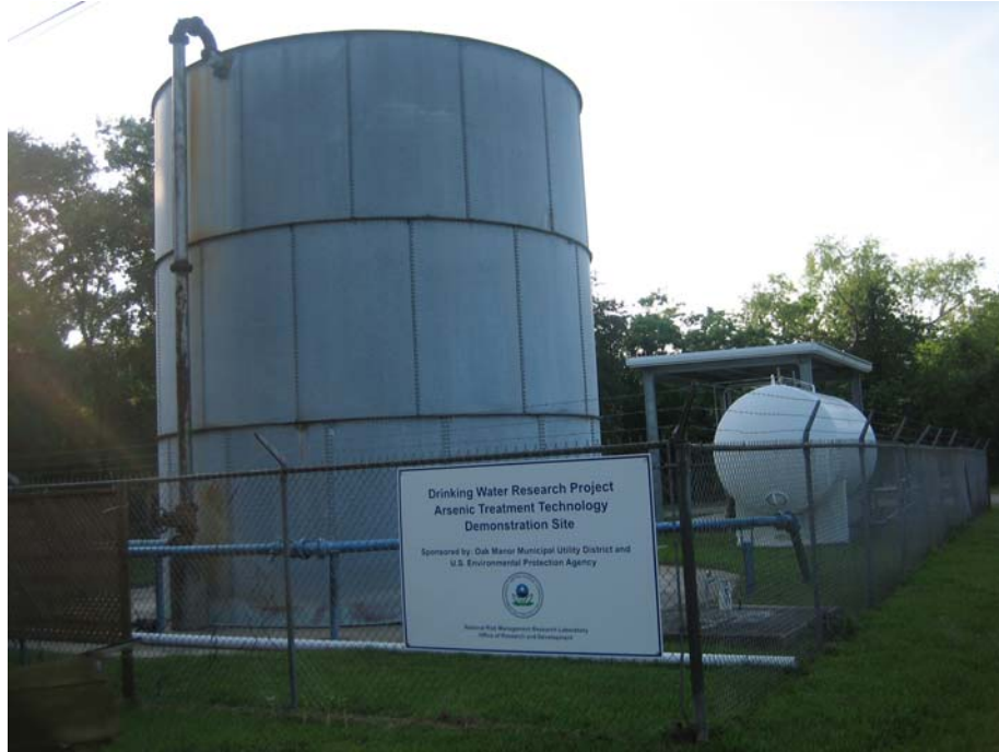
Figure 4-2. Preexisting Storage Tank (in Foreground) and Hydropneumatic Tank (in Background)
