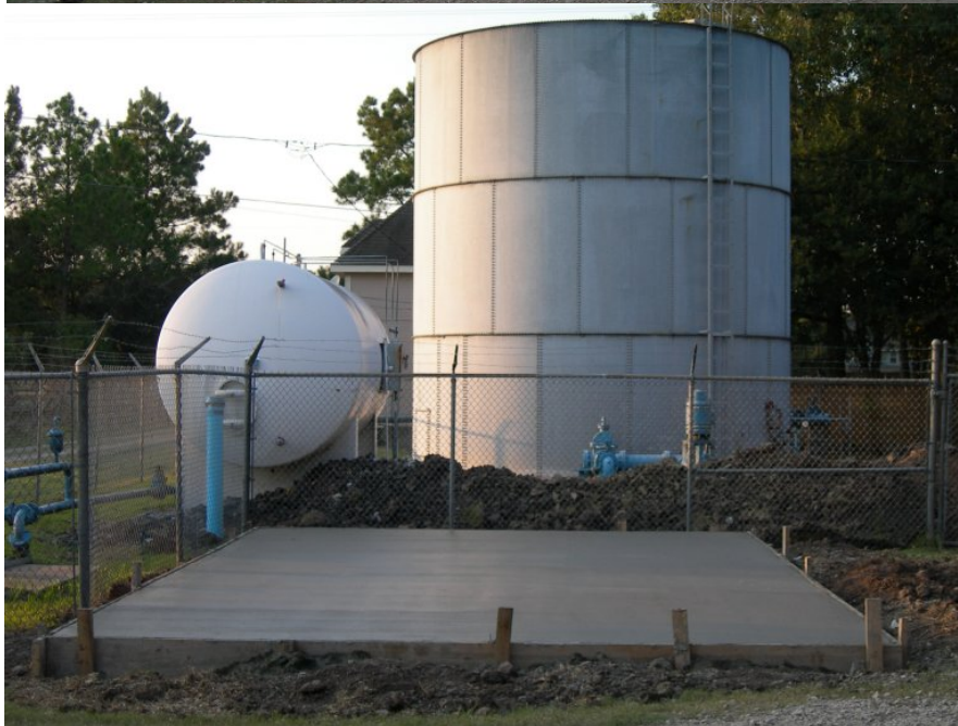
Figure 4-11. Construction of Concrete Pad with Storage Tank and Hydropneumatic Tank (in Background)
