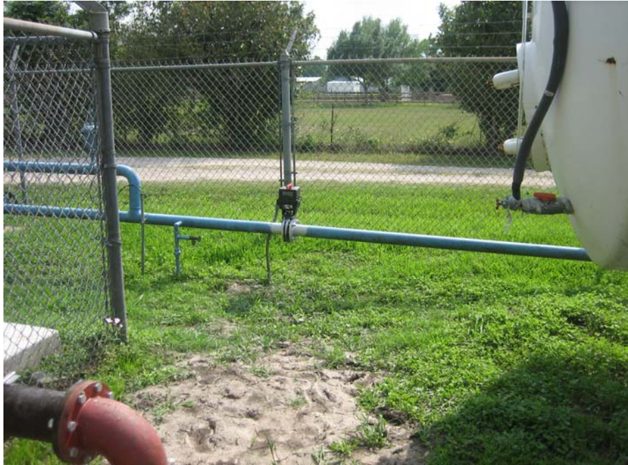
Figure 4-9. Valve MB-127 to Supply Additional Treated Water from Hydropneumatic Tank During Backwash
