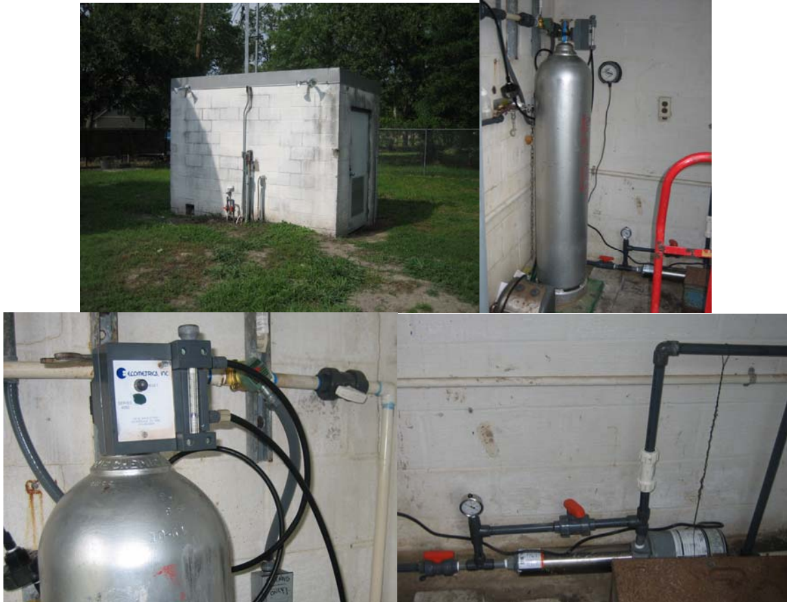
Figure 4-7. Gas Chlorination System (Clockwise from the Top: Shed Housing Gas Chlorination System, Gas Cylinder, Chlorine Ejector, and Chlorinator Unit)
