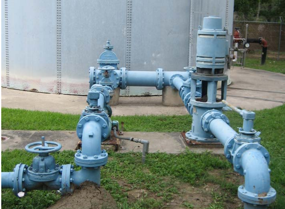
Figure 4-4. Booster Pumps and Entry Piping to Distribution System
