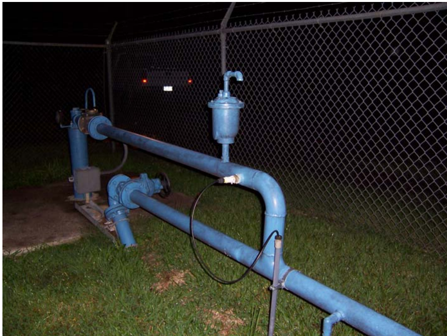
Figure 4-3. Preexisting Polyphosphate Addition Point
