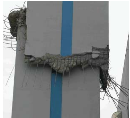
Details of failure of reinforced concrete at the Kashiwazaki municipal incinerator.
