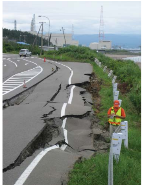
Coastal damage adjacent to the Kashiwazaki-Kariwa Nuclear Power Station.
