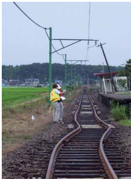
Permanent lateral deformation of train tracks at the Arahama station, the result of compression due to surface waves.
