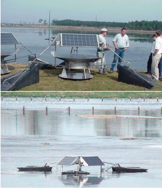
Figure 7. SolarBee® installed in City of Myrtle Beach, South Carolina, 50-acre wastewater lagoon.
