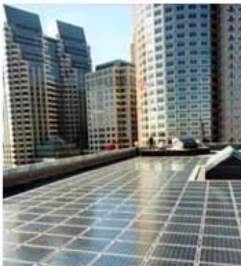
Figure 1. Solar panels (or arrays) on the roofs of buildings.
