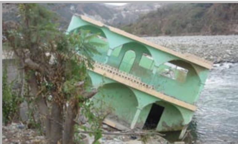
Hurricane Stan destroyed this building and many other structures in Central America and Mexico during the 2005 hurricane season, the most active on record.
