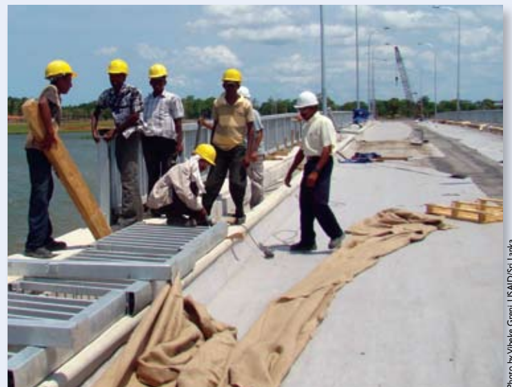
Five formerly unemployed and unskilled local young men on the bridge where they worked placing steel works, handrails, and concrete deck panels. They now have the skills to pursue future jobs in construction.
