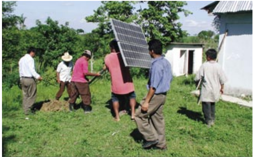
A home in Veracruz, Mexico, obtains solar power as a result of decade-long collaboration on energy projects between USAID and the U.S. Department of Energy's Sandia National Laboratory.
