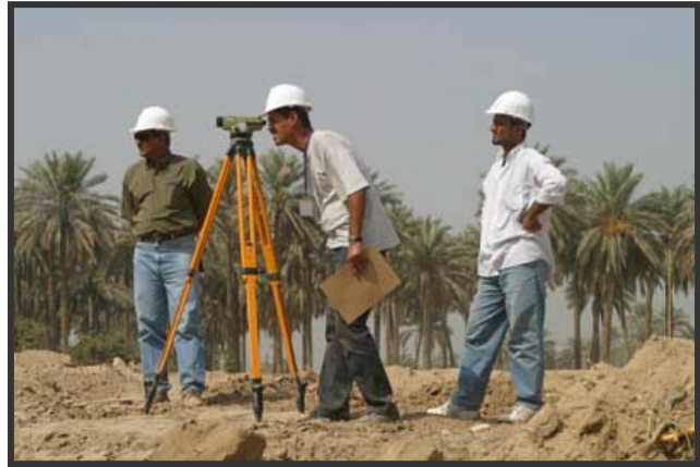
Iraqi civil engineers, survey the site preparation for an extension to the Saba Nissan water Treatment to expand drinking water for the Baghdad region. (Photo: Thomas Hartwell)
