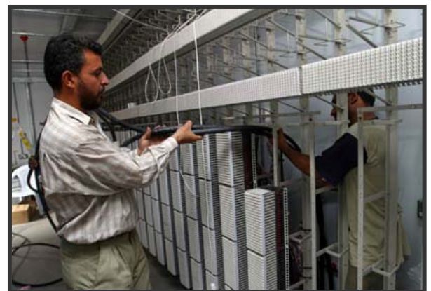
The Al-Mamoun Telephone Exchange where repair work will restore telephone services to approximately 30,000 subscribers. (Thomas Hartwell)
