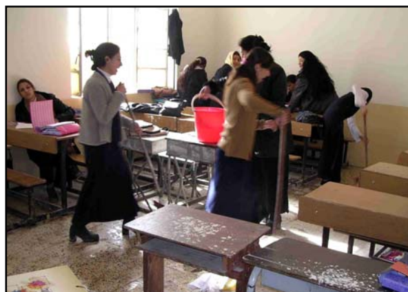
Community members in Baghdad's Karada District rehabilitated Al Sharkiyah Technical School for Girls. Photo: USAID
