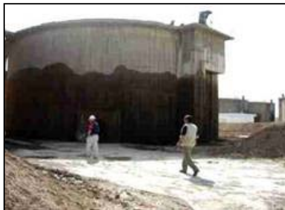
Kerkh digester tank with diesel-stained walls. Photo: USAID
