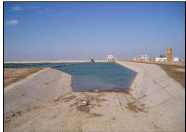
The renovation of the Sweet Water Canal's sediment retention reservoir system—a three-month effort—is nearly finished. Photo: USAID
