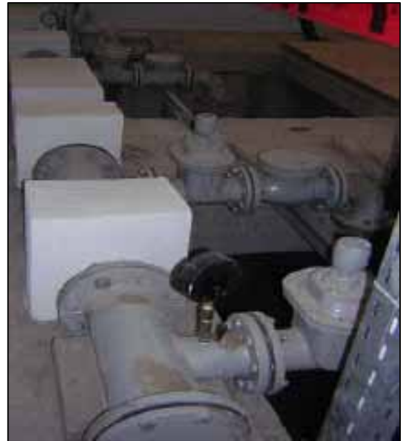
When complete, repairs to a sewage system in a north Baghdad suburb will improve service to 1.5 million people.
