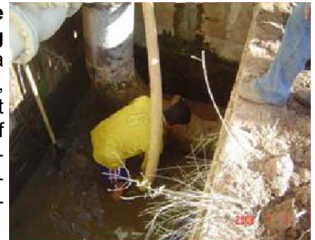
USAID partners replaced the old, cracked asbestos pipe lines, improving water quality and delivery.
