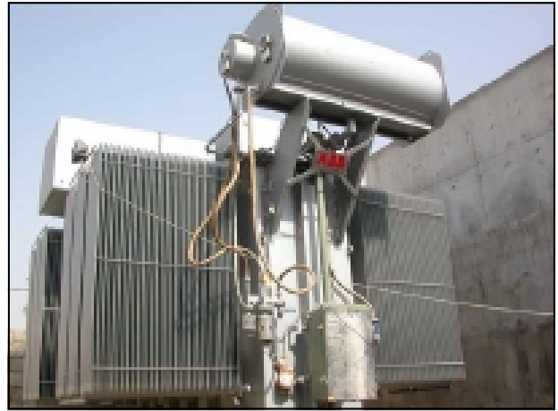
Substation transformer and coolant oil tank
