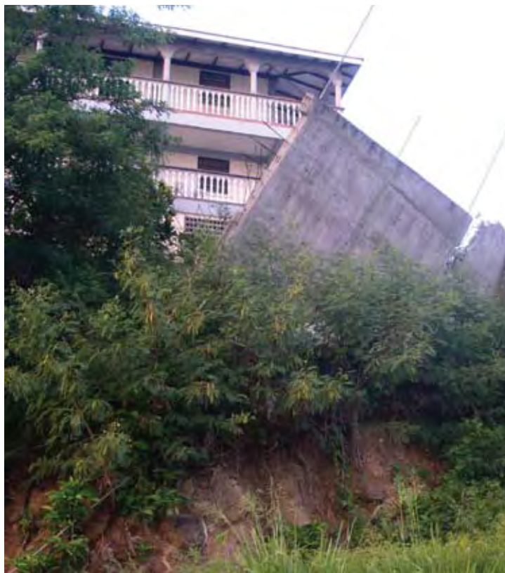
A large slab of concrete from a damaged building rests precariously on a hilltop in Dominica following Hurricane Dean (Photo by Julie Leonard, USAID).
