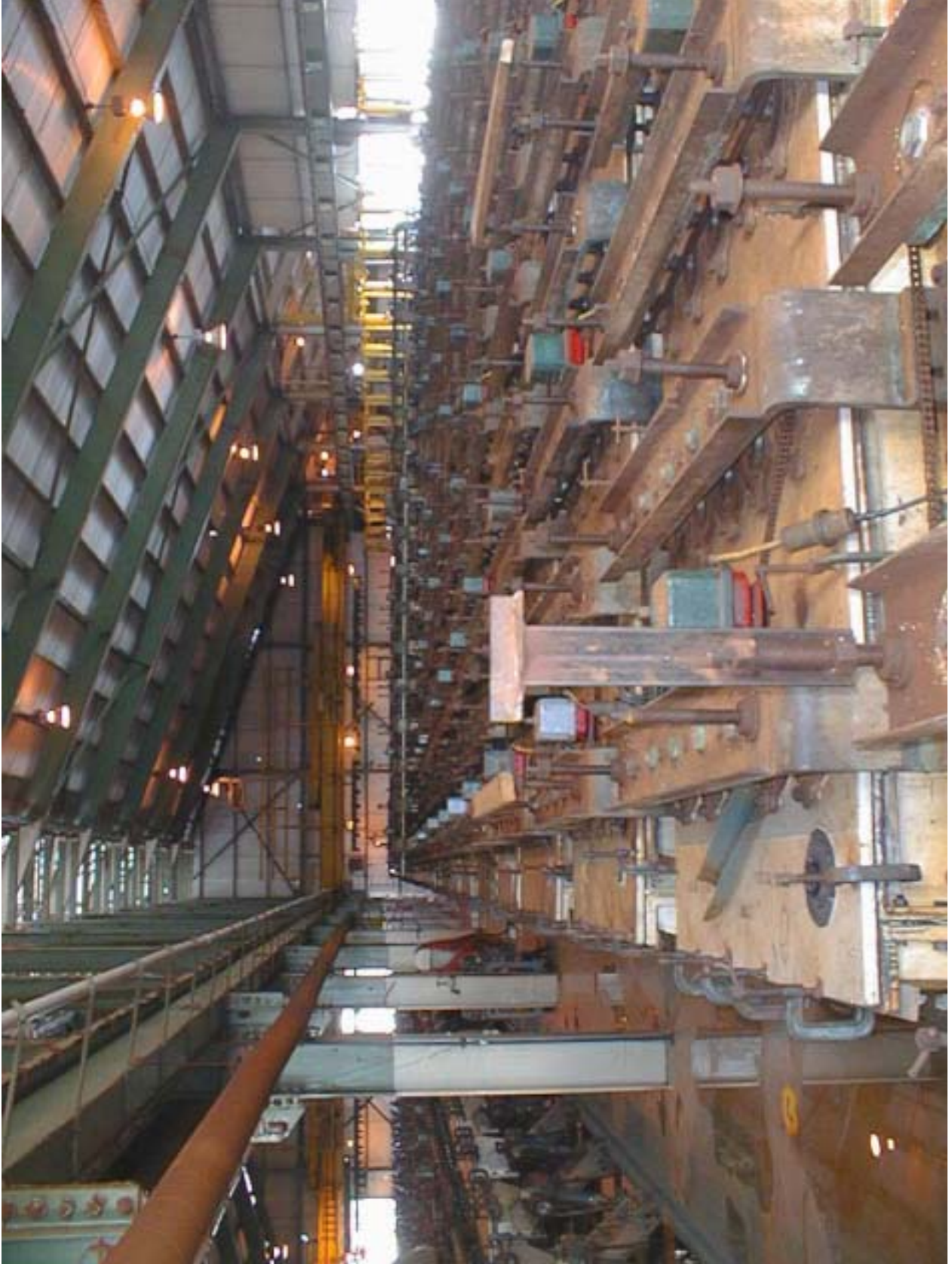
Figure 3-6. North line of electrolytic cells in Olin cell building.
