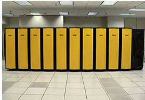
Ten racks of XT3 containing nearly 1,000 AMD Opteron processors stand side-by-side in PSC's machine room at the Westinghouse Energy Center, Monroeville, PA.
