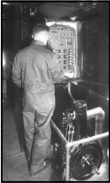
Switchboard and lighting plant on Car No. 3.
