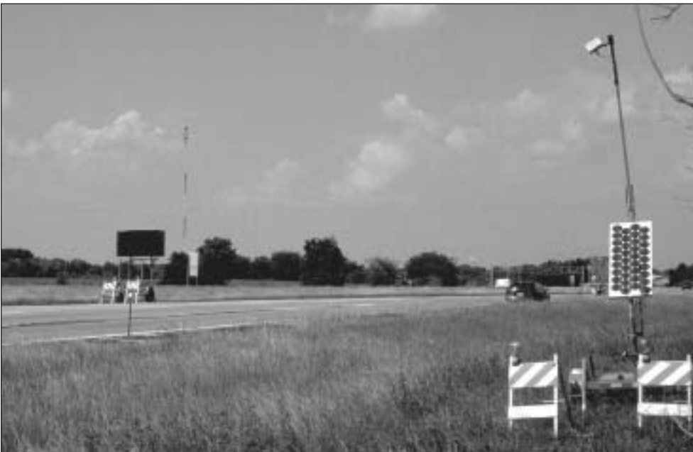
Figure 2 – Some of the I-55 System Components: DMS, and Traffic Sensor with Solar Array
