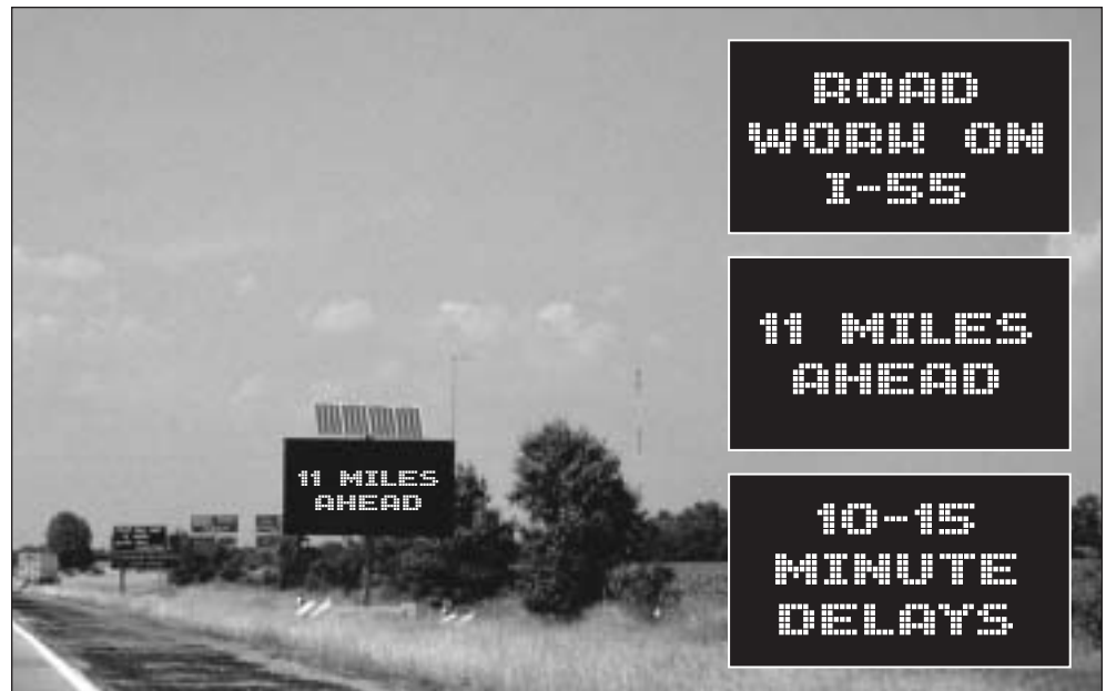
Figure 5 – DMSs Alerted Drivers to Traffic Conditions in the I-55 Work Zone (Figure Shows an Example 3-Phase Message)
