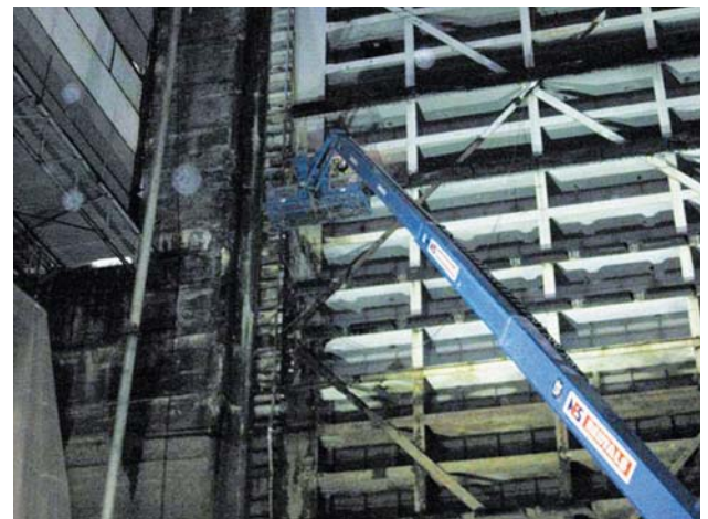
Crews being lifted to replace damaged rubber fenders on the downstream miter gate.
