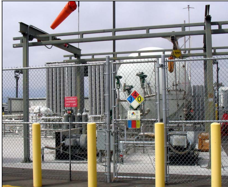
Figure 20. Liquid Hydrogen Storage Tank and Vaporizer
