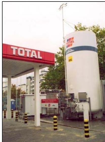
Figure 25. Liquid Hydrogen Storage Station
