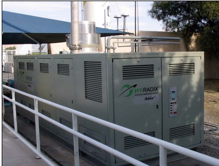
Figure 21. Natural Gas Reformer
