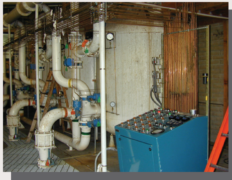
Water supply sand filter and control box — Warm Spring NFH, OR. USFWS photo.
