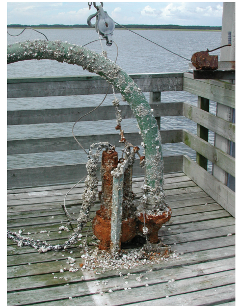
Corroded saltwater pump station — Bears Bluff NFH, SC. USFWS Photo.
