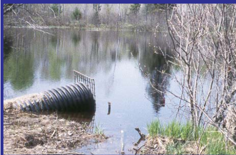
This culvert on Hardwood Creek in Michigan was too small and dark to allow fish to pass under this road (upper). The culvert was replaced with a new structure (below) using funds from partners and the Fish Passage Program.
