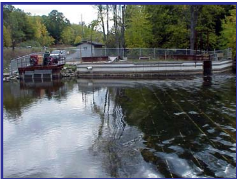
-GLFC The electrical barrier on the Pere Marquette River is energized when adult sea lampreys migrate into this Great Lake tributary to spawn. The series of electrodes can be seen below the water surface.
