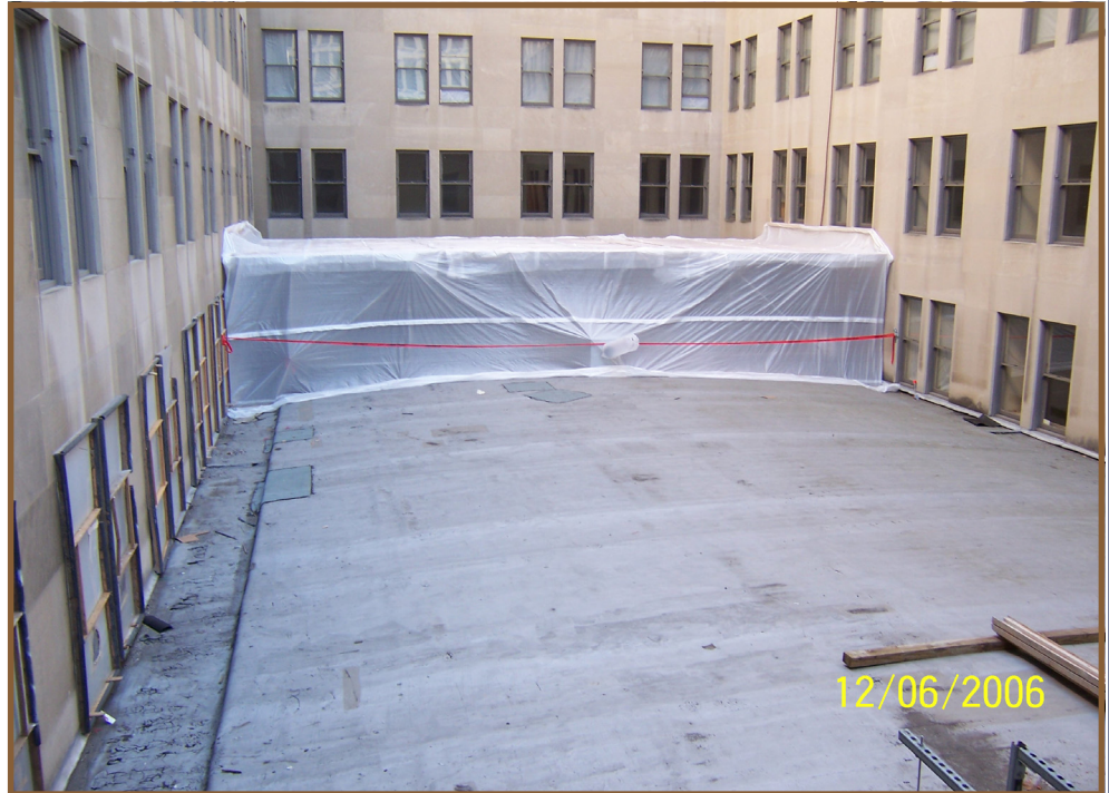
The gym roof demolition will re-introduce skylights that were a part of the original gymnasium when the building was completed in 1935. A temporary shelter will be used while work is being completed.
