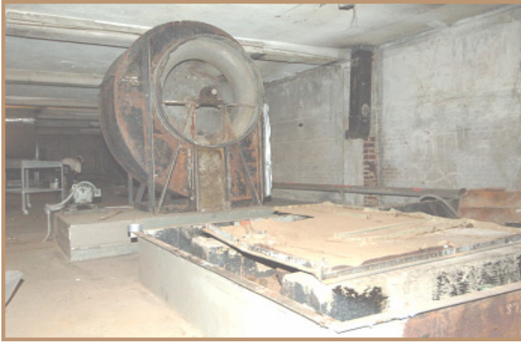
An original building fan stands approximately 8 feet high on the M floor/ This was part of the first centralized heating, ventilating and air conditioning system in a large federal building. This is being replaced with modern equipment in a more efficient HVAC system.
