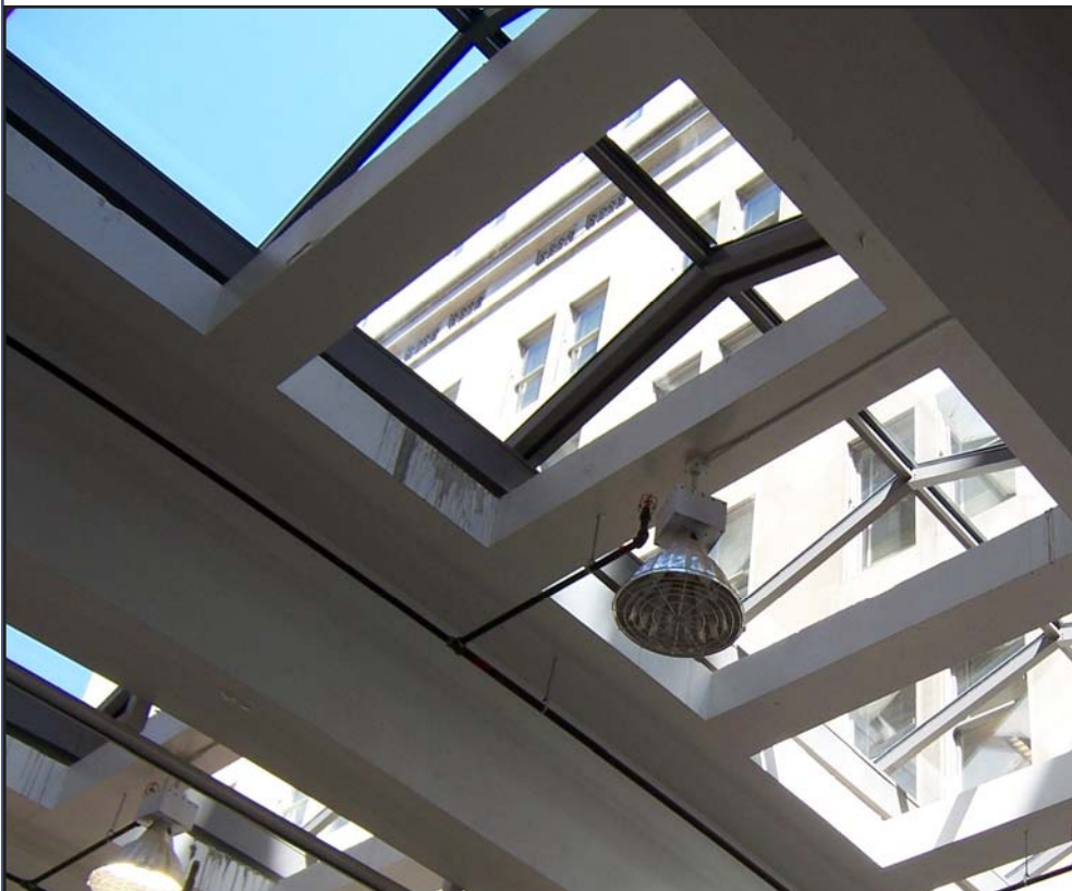
The gymnasium opens in September with a new floor and new skylights.
