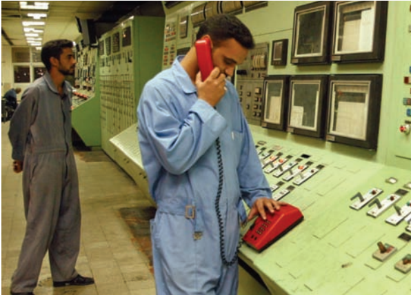
Iraqi engineers monitor controls at the Baghdad South power plant. IRRF funds are helping to repair Iraq's nationwide electrical system.
