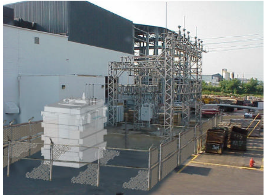
5/10-MVA Transformer at WES Plant
