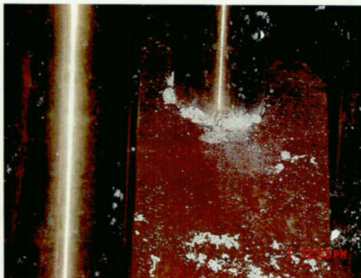
Figure 1 – Typical Boric Acid Accumulation Around a Failed CRDM
