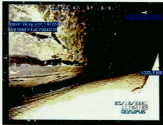
Figure 7 – Insulation Gap at Penetration #59
