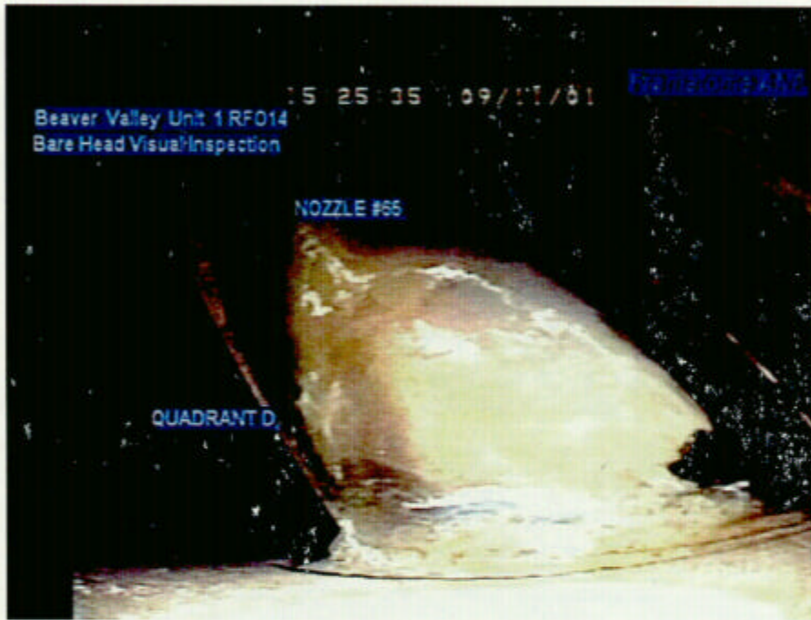
Figure 9 – Penetration #65 Corrosion at Base of Penetration
