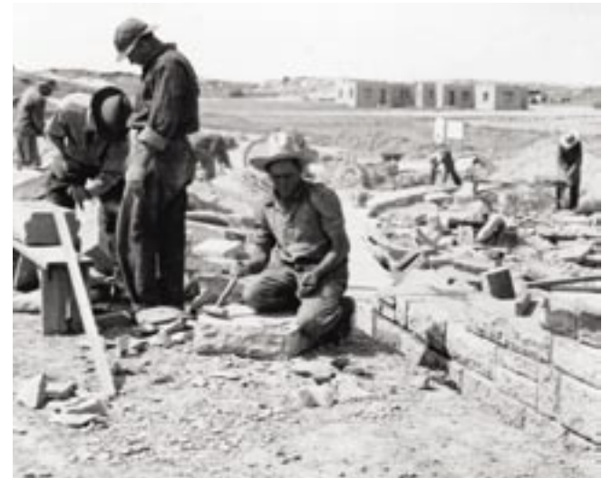
Construction of site walls near Rainbow Forest Headquarters, early 1930s. PEFO Photo Archive #15588
