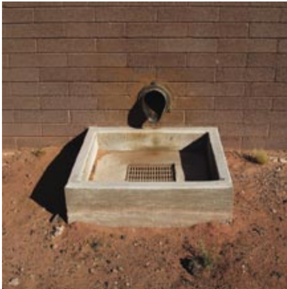
This water removal system, implemented on the Maintenance building, is well designed. Unsightly downspouts have been eliminated, the materials and components are durable and handsome, and the system was carefully inserted into the building. 2004 photo by author
