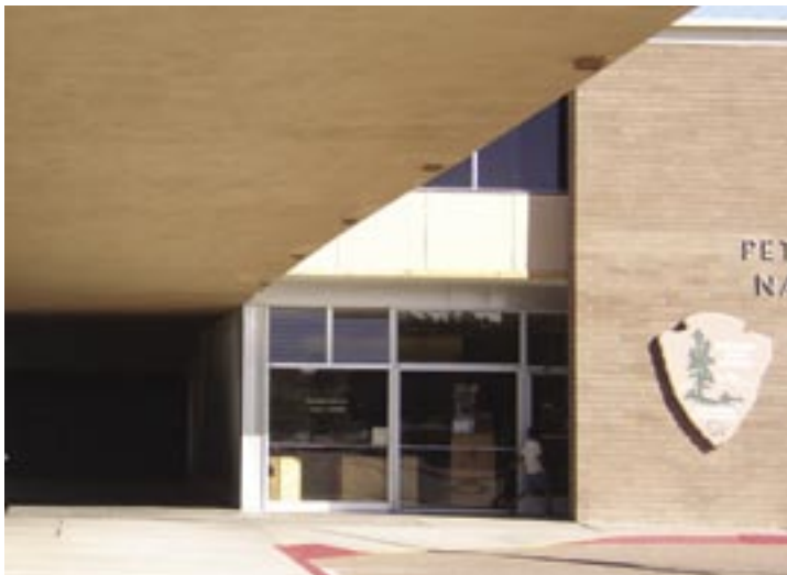
Aluminum storefront systems hold up very well with proper maintenance and cleaning. 2004 Photo by author
