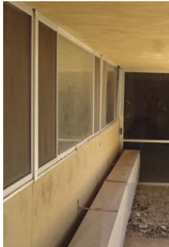
Often it is the case that it isn't the failure of the window itself that is the problem at the PDCCHD, but the failure of the window due to shifting soil conditions. 2004 Photo by author
