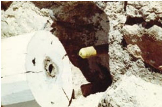
The viga end has been removed and a threaded rod has been set with epoxy into the existing viga. Note how viga end was removed just below the surface of the wall.
