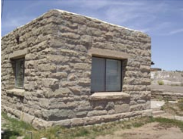
The color of the mortar should match the color of the original mortar. The use of gray mortar, as seen in the repointing of RF unit 52-C should be discontinued. Photo by author
