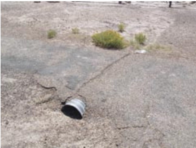
Culverts should be integrated into trails with installation appropriate to prevent tripping and provide aesthetic appeal. This exposed ends of this culvert make it more obtrusive than necessary. Photo by author
