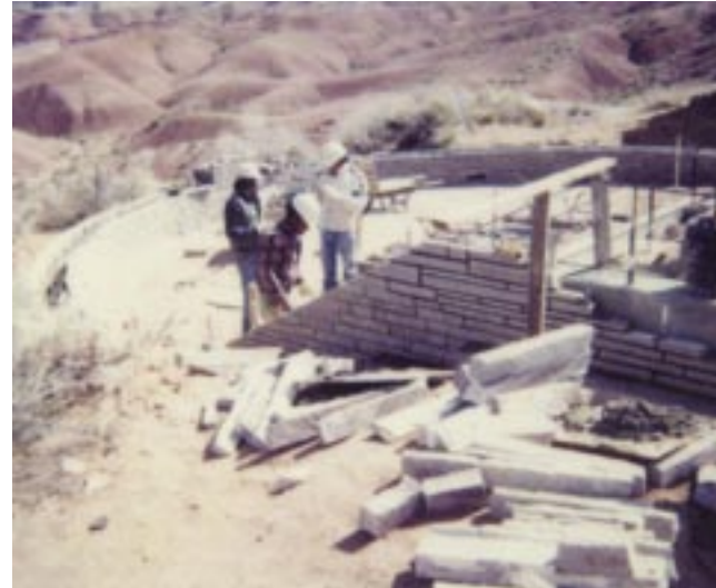
This construction photo from Tiponi Point shows stone being used as a veneer over a concrete wall. This construction system is still widely used throughout the park and is appropriate for new construction. PEFO Photo Archive
