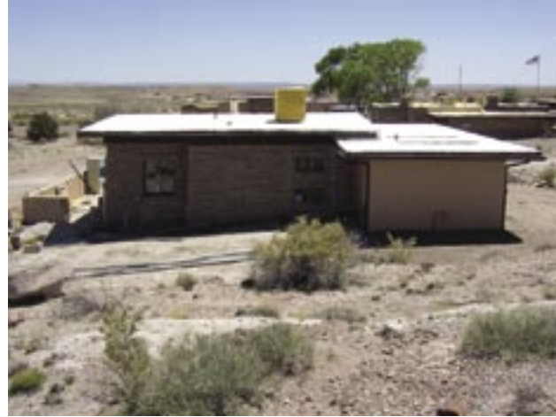
The glaring white color of this roof is inappropriate. A better color choice would be tan or a color that helps to blend the roof with the distant landscape
