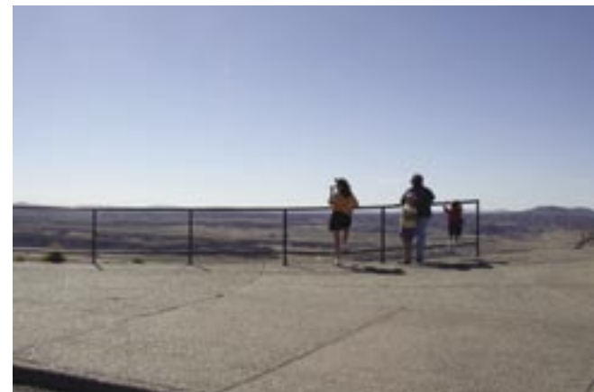
This railing along the parking area at Pintado Point is susceptible to damage by vehicles and visitors and could be replaced with a low stone wall. Photo by author
