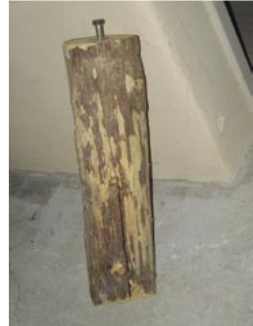
New viga end showing receptacle for receiving threaded rod. In this case, receptacle is being protected from damage with a bolt before installation. Photo by author
