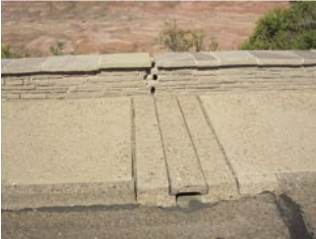
Draining water under this landscape wall at the “no-name” turnout likely caused the crack in the wall to develop from movement in the soil. Photo by author
