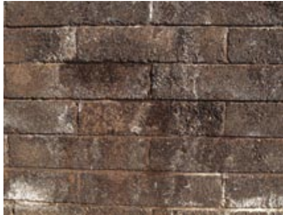
Efflorescence and deterioration caused by a sprinkler. See National Park Service Preservation Brief 1 for efflorescence removal information. 2004 photo by Author
