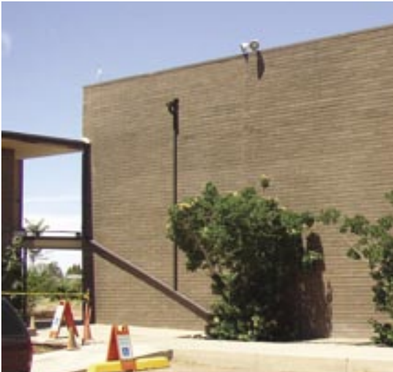
Because the Petrified Forest Community Complex was designed only using right angles, this downspout configuration looks especially out of place. 2004 photo by author
