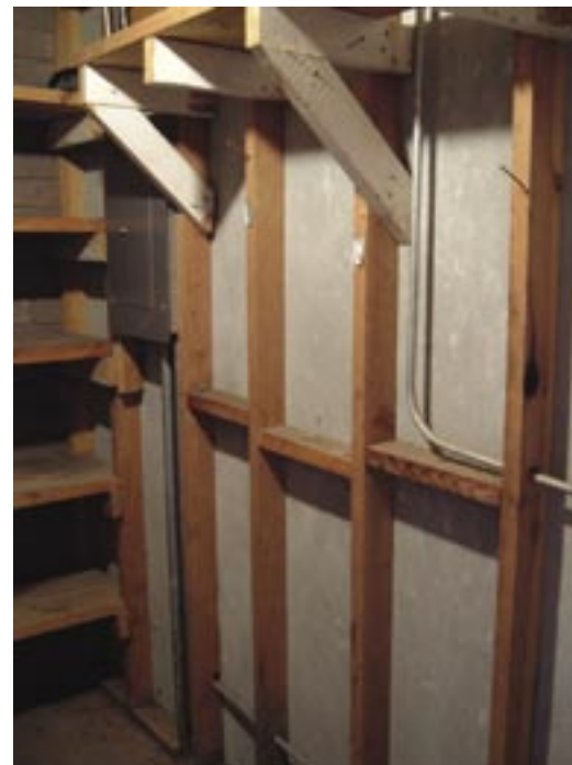
It is likely that wall panels used in the Painted Desert carports and gatehouse contain asbestos. 2004 Photo by author
