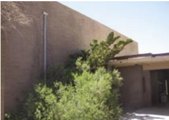
There are two problems with this downspout. One, it should be painted to better blend with the surrounding buildings. Two, there is an broken seal where the downspout leaves the roof that is causing damage to the wall beneath . 2004 photo by author
