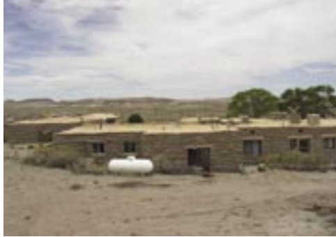
Because of the change in elevation at Rainbow Forest, many roof tops can be seen from public areas. New roofs should blend with the sandstone color of the walls and surrounding landscape, as best as possible. Photo by author
