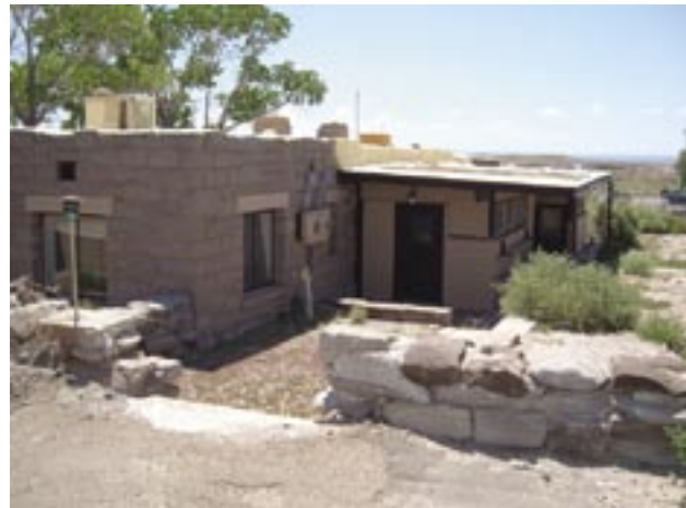
Foam roofing applied to the parapets and walls of buildings at Rainbow Forest should be removed carefully and with the assistance of an experienced professional. See Sandstone Masonry Cut Sheets for more info. Photo by author
