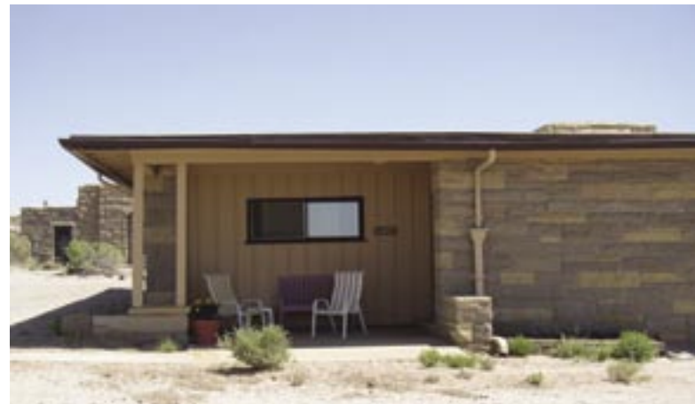
This downspout at Rainbow Forest complements the building it is serving well, but where is the water going? 2004 photo by author
