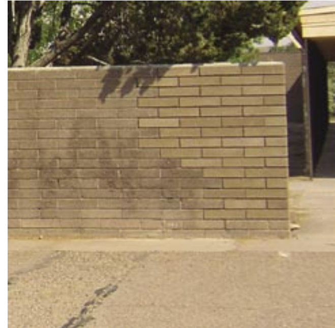
Inappropriate repair. Replacement block is randomly "toothed" into existing wall. Color and texture of the new block is emphasized by random replacement pattern. A more distinct separation, including a control joint, should exist between new block and the historic block.
