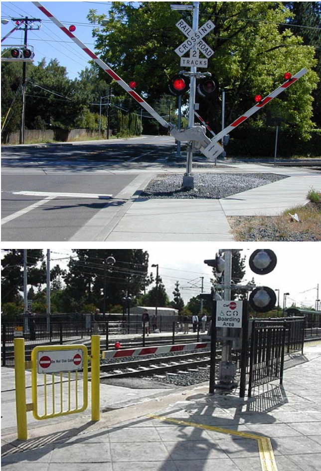
Figure 76. Pedestrian Automatic Gate Examples
