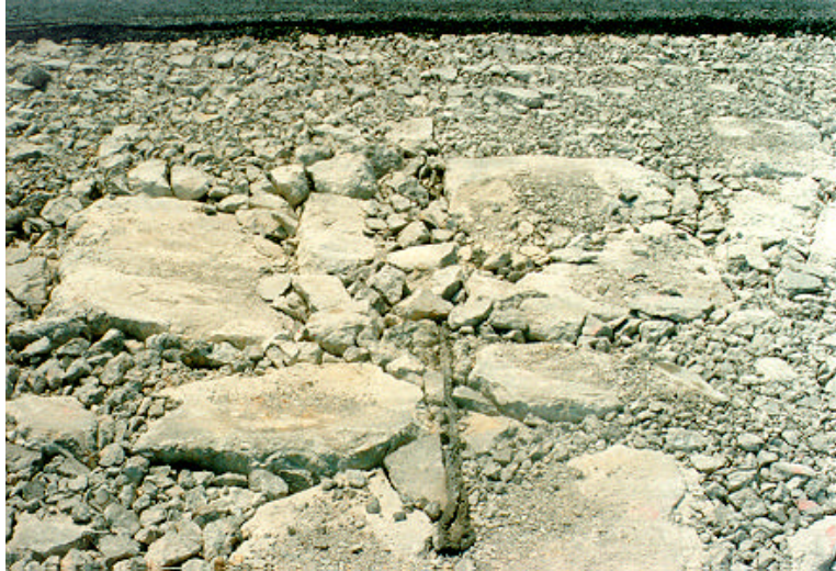
Figure 12. Large Rubblized Pieces (IL 38 1994).
