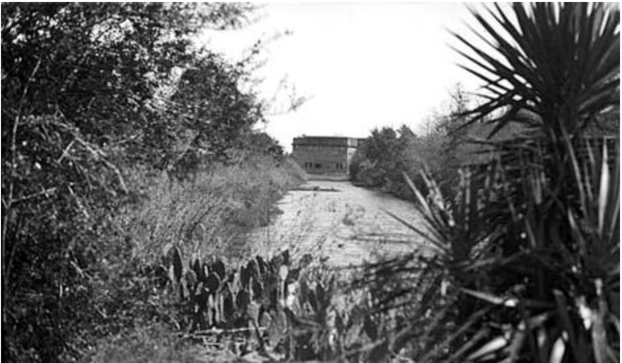
FIGURE 7. View on top of fort terreplein before restoration work, HABS photo, c. 1930
