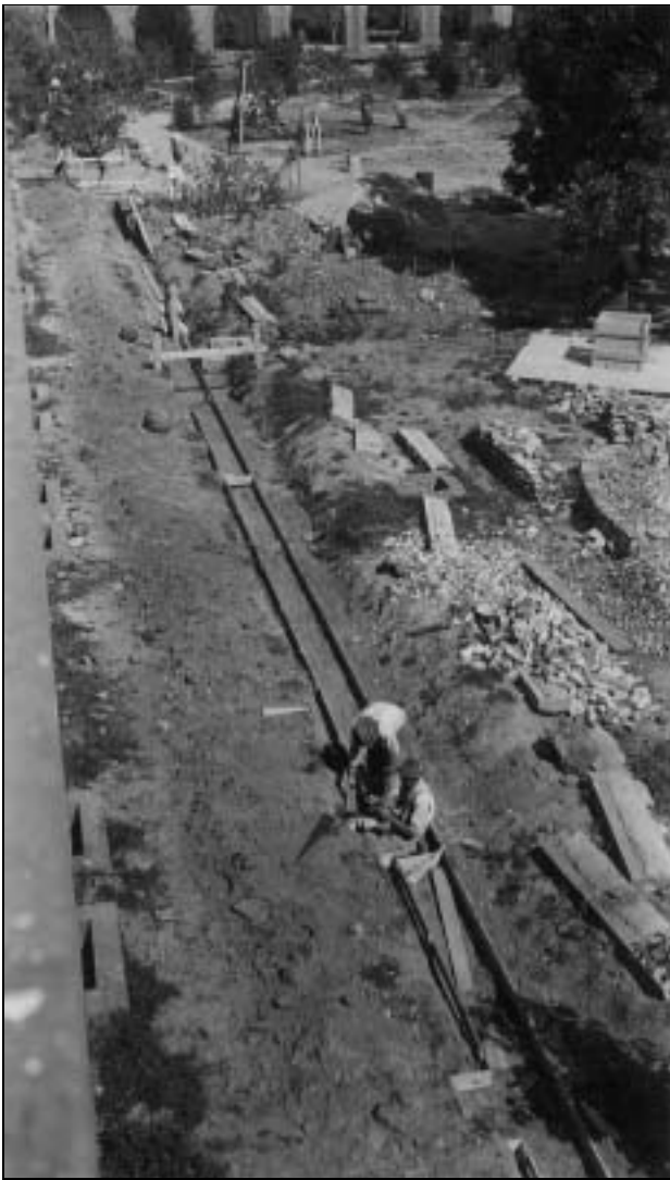
FIGURE 10. CCC enrollees place concrete footings in parade ground for gorge sidewalk construction, October 1934
