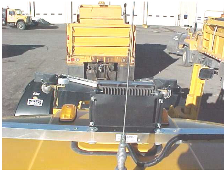
Figure 15: Eaton VORAD Radar Antenna Installed on ADOT Plow
