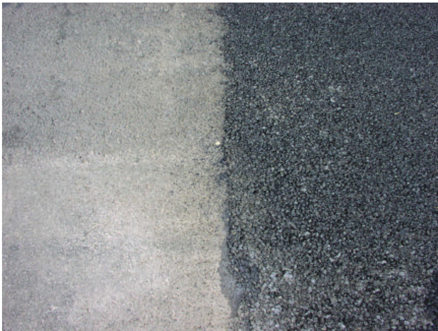
Figure 6. SMA on Left Adjoining PFC on Right
