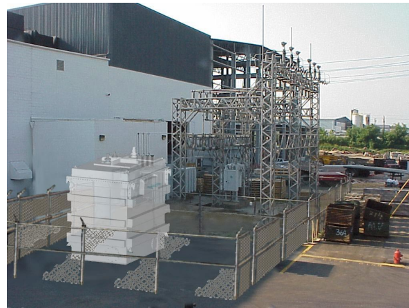
Fig. 2.31. The 5/10-MVA transformer in planned location at WES factory.
