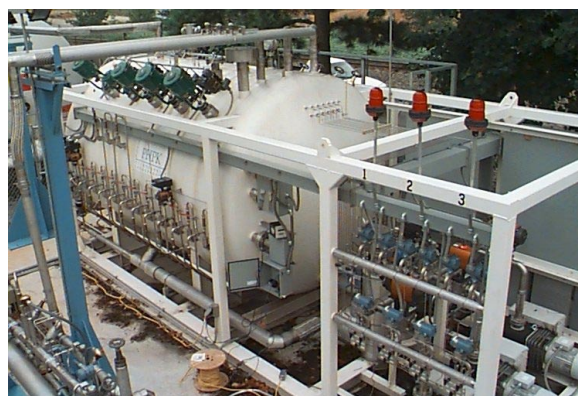
Fig. 2.21. HTS power cable cryogenic system.
