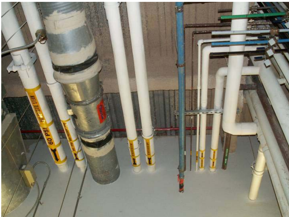
Photo A-4 Service Bay
