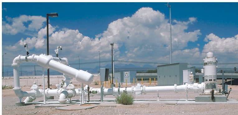
This typical artificial recharge well has the dual function of pumping and injecting. (The tall object on the far right is the electric motor for the pump).
