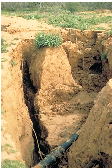
A natural-gas pipeline undercut by an earth fissure was exposed through erosional widening of the fissure. The pipeline was evacuated and cut to determine the stresses on it. Tension was evident, but no shear.
